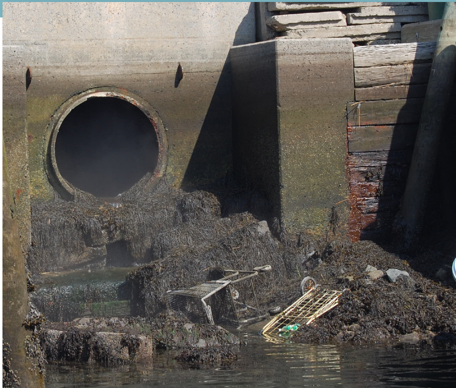
CSO discharge point on the Portland waterfront, adjacent to the Casco Bay Ferry Terminal.
