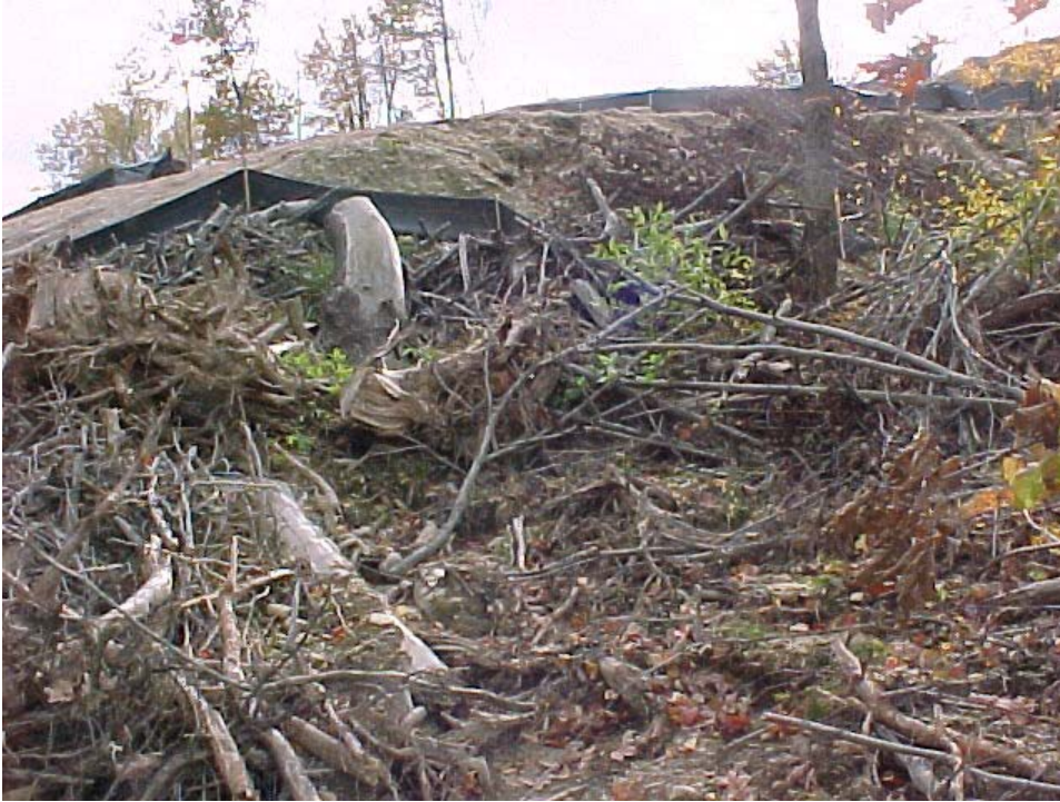
Figure 6: Erosion gully in poorly stabilized soil
