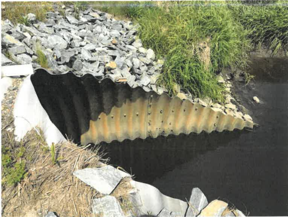
Photo 2 (06-20-18): Submerged inlet of 10.5-foot wide by 11.5-foot tall corrugated aluminum elliptical pipe with flared end and rip rap headwall on east side of Sawyer Road. Additional headwall rip rap should be added to the headwall.
