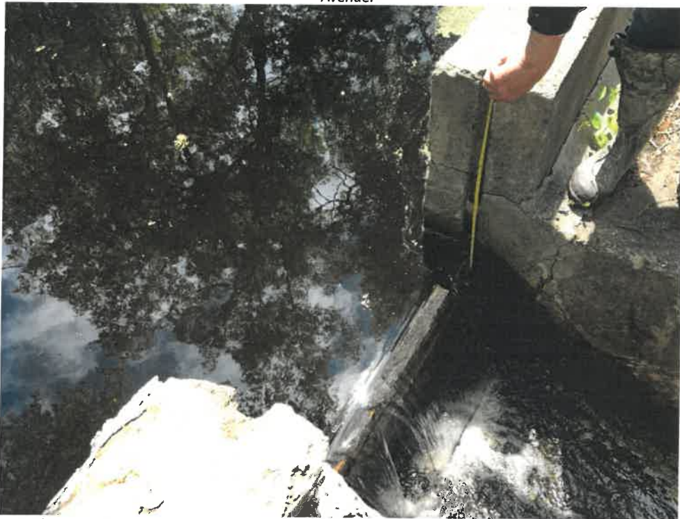
Photo 4 (06-06-18): Closeup view of adjustable elevation wooden board weir outlet to pond impoundment on the south side of Spurwink Avenue.
