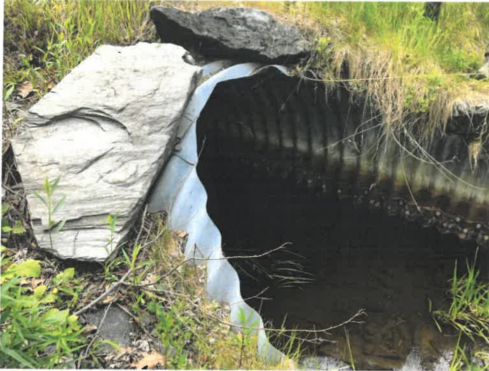
Photo 6 (06-06-18): Looking at the submerged outlet of 8 foot, 2-inch-wide by 5 foot, 9-inch-high steel plate pipe arch cross pipe. Rip rap stones are sparse, but provide a headwall.
