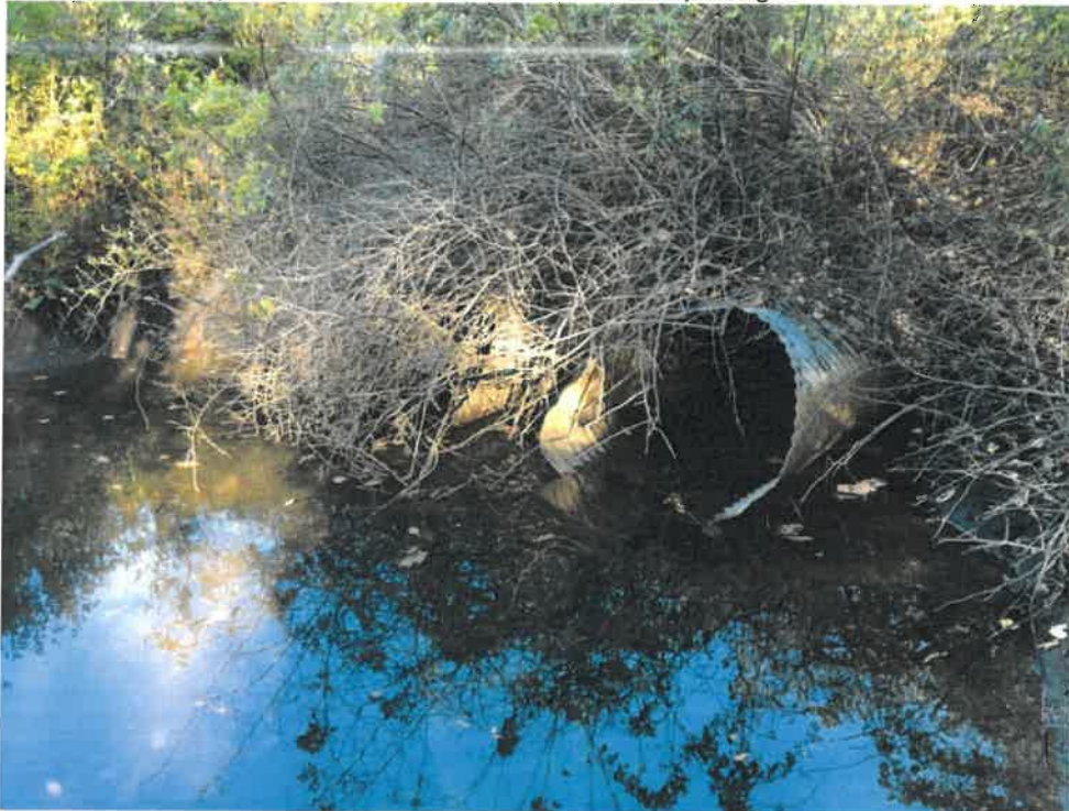
Photo 6 (10-22-18): One of the outlets of the culverts on the south side of the embankment is obscured by vegetation and partially buried in sediment. Outlet has some stone in the channel, but no formal plunge pool or visible headwall.
