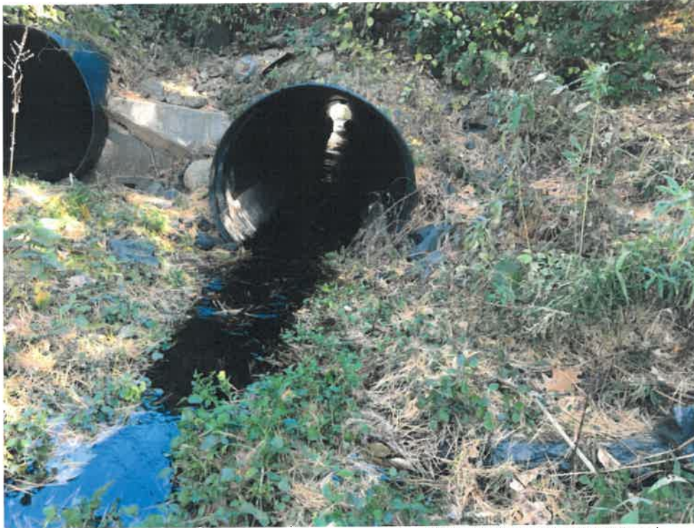
Photo 3 (10-22-18): Looking northerly through the inlet of one of the two 48-inch high density polyethylene liner pipes within the original corrugated aluminum cross pipes. The invert of the main carrying pipe is lined with a corrugated metal pipe section to reduce the velocity of flow through the pipe.
