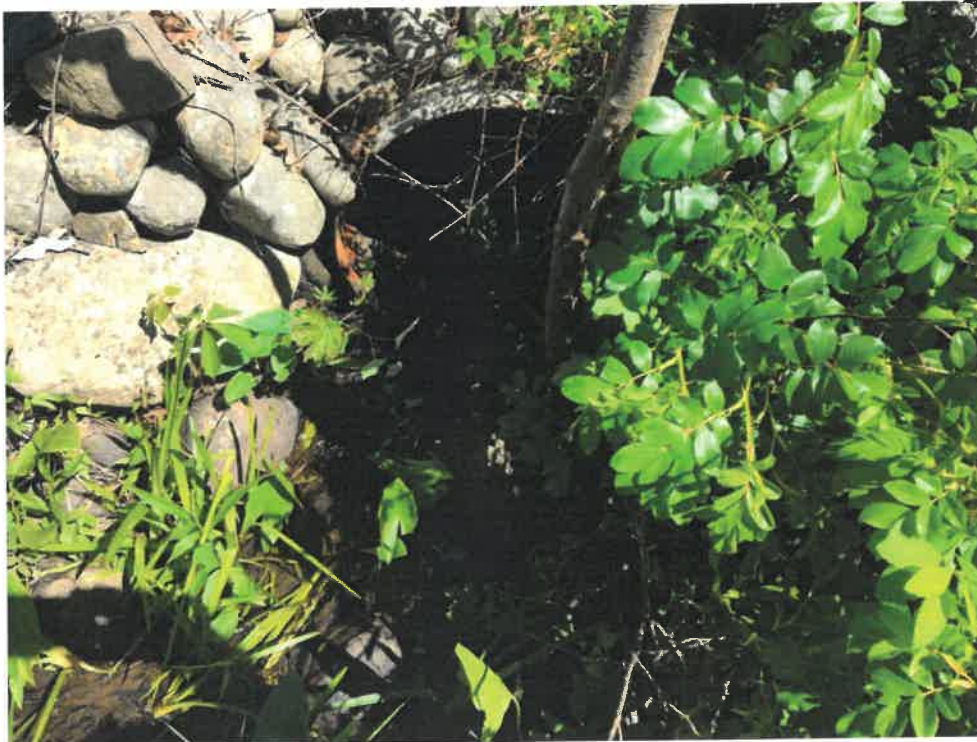
Photo 2 (06-06-18): Inlet of 24-inch corrugated aluminum cross pipe with a rip rap creating a headwall and apron. Inlet is on the west side of Spurwink Avenue and very thick vegetation made locating the culvert difficult.
