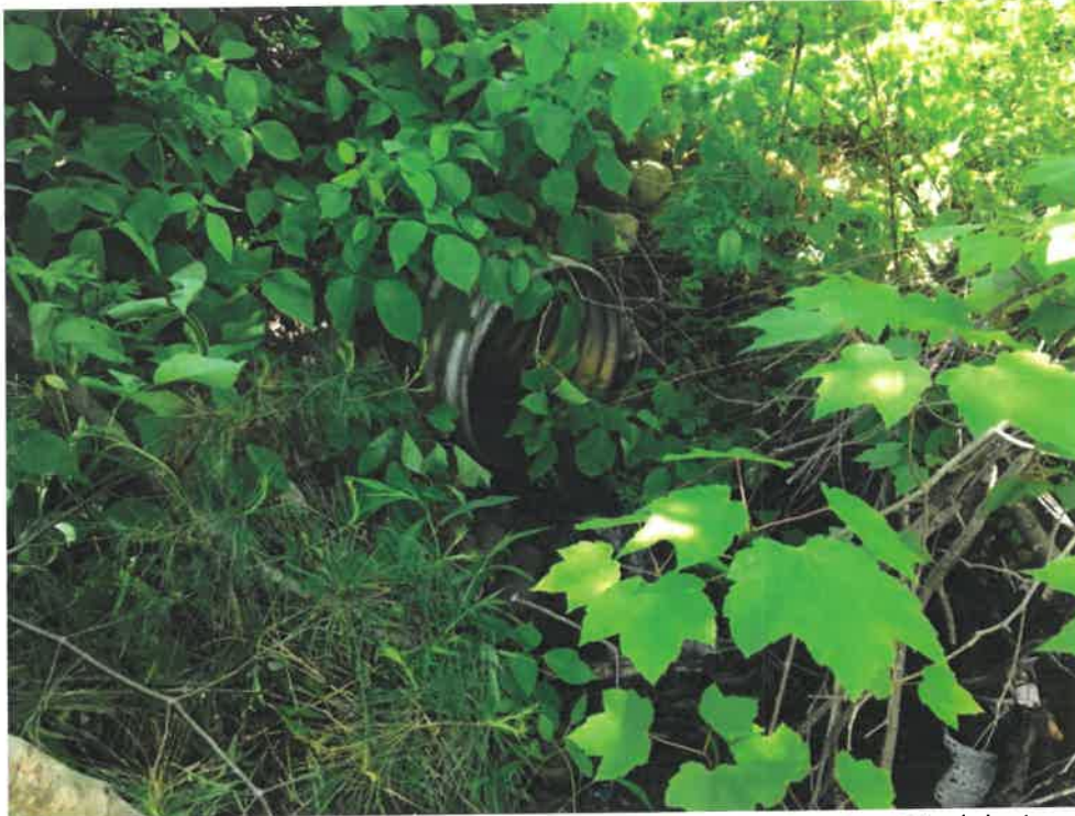
Photos 3 (06-06-18): Hanging culvert outlet on east side of Shore Road of the 24-inch corrugated aluminum pipe.
