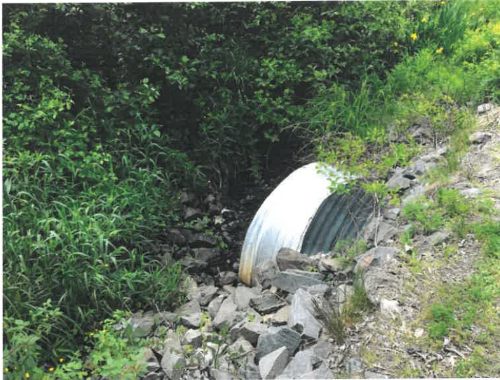
Photos 3 (06-06-18): Culvert inlet on west side of Spurwink Avenue is submerged within the corrugated aluminum pipe. Upstream vegetation obscured channel at the time of the photo.
