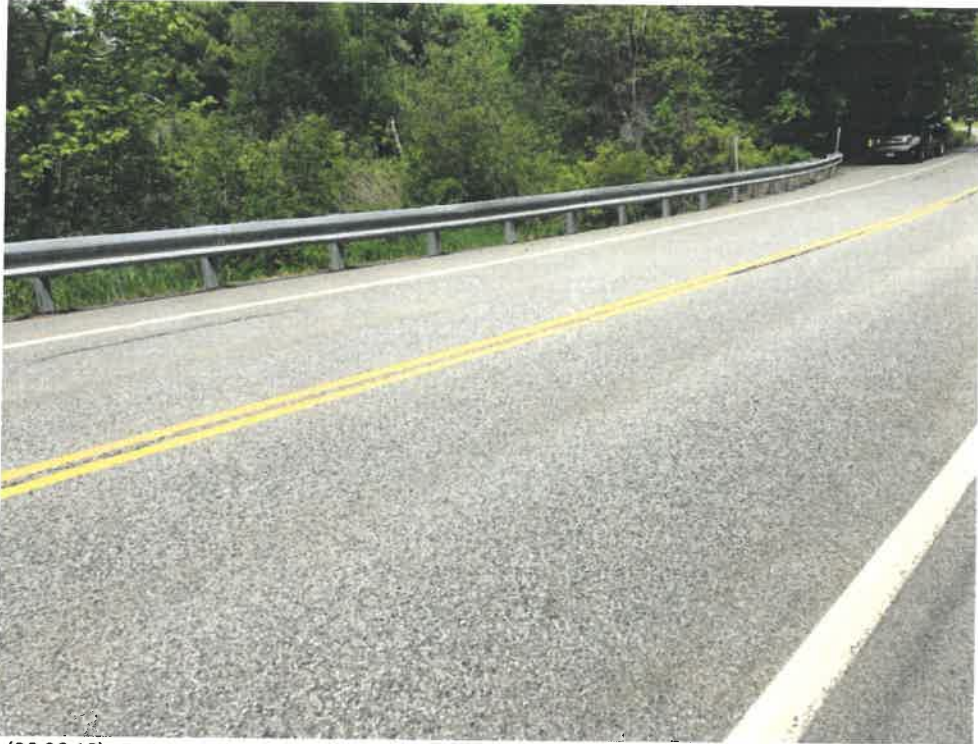
Photo 1 (06-06-18): Facing north at the surface of Spurwink Avenue at the crossing of the pond outlet pipe/culvert that discharges into Pollack Brook.
