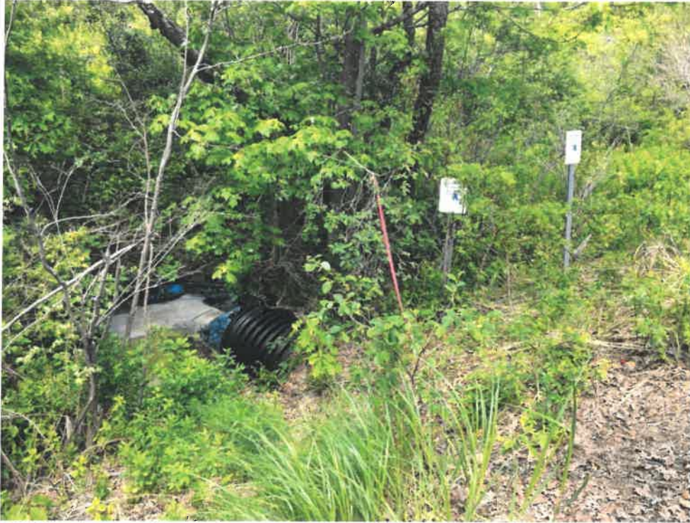
Photo 7 (06-06-18): Looking north down the Spurwink Avenue embankment at the outlet of the 36-inch HDPE culvert on the north side of Spurwink Avenue. Signs indicate the presence of the National Wildlife Preserve with the pink flagging tied to a survey pin.
