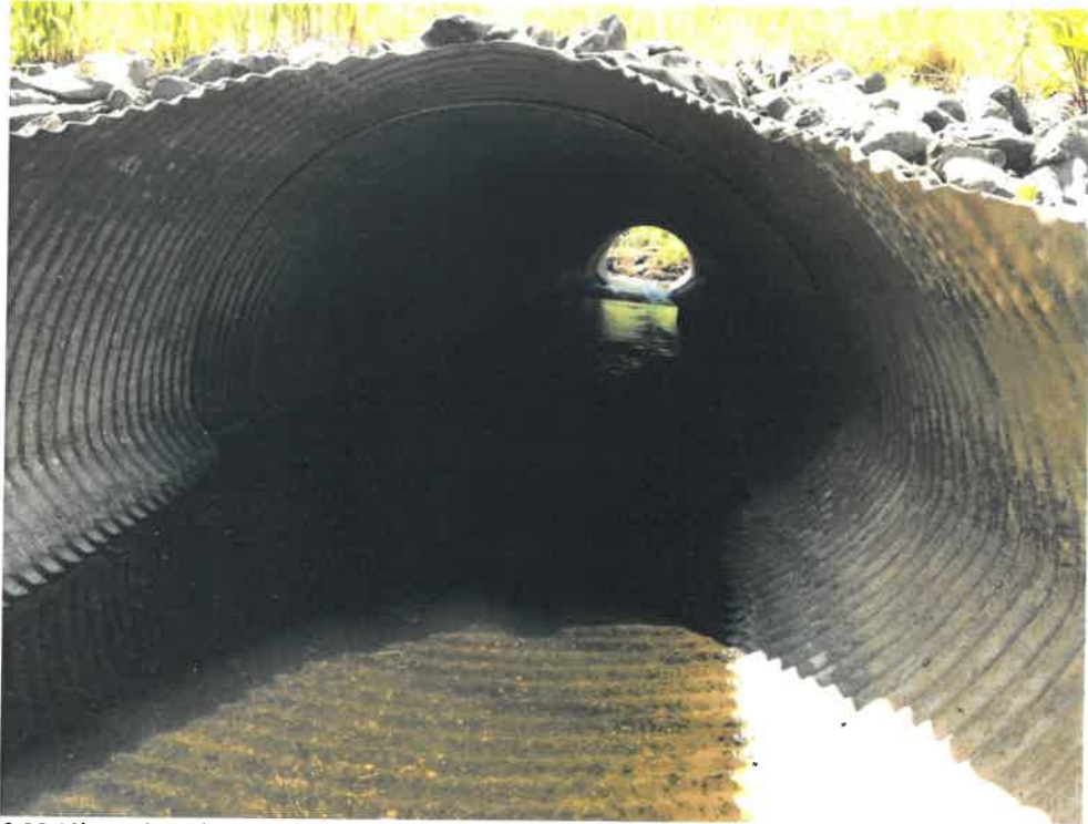
Photos 3 (06-06-18): Looking through the culvert from the inlet side, interior of the elliptical pipe appears visually to be in good condition, however, the flared end section appears to be pulling away from the last section of pipe.
