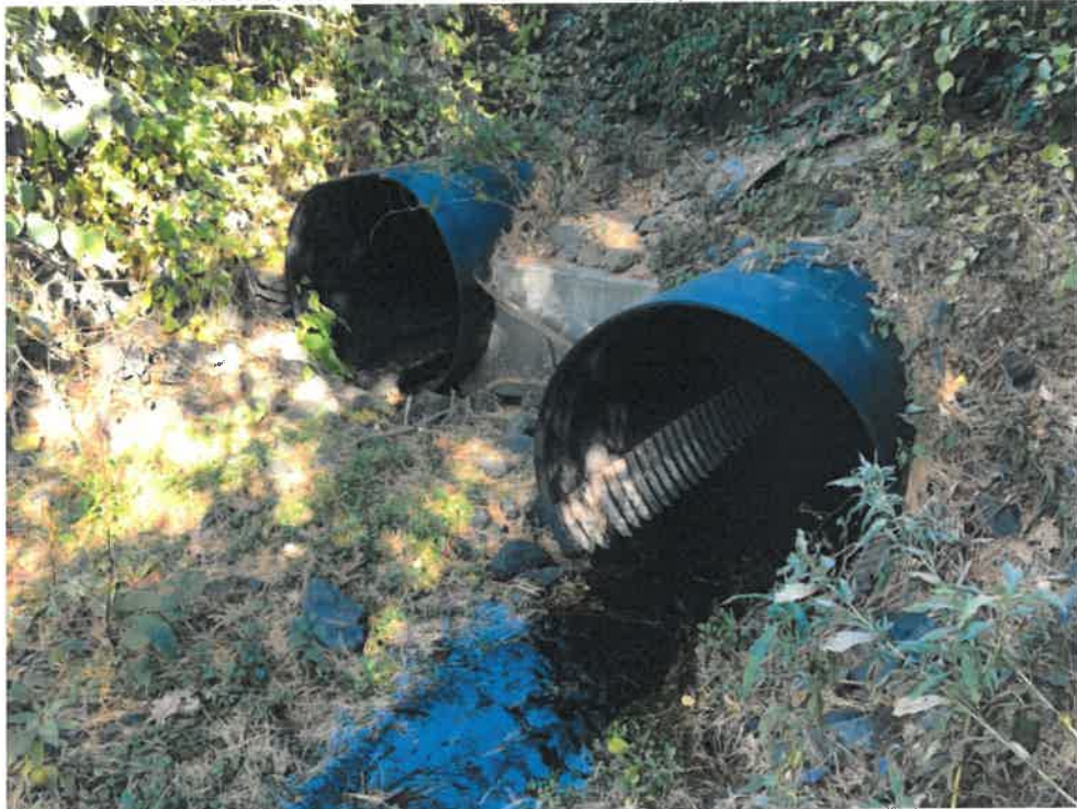
Photo 2 (10-22-18): Inlet of two 48-inch high density polyethylene liner pipes within the original corrugated aluminum cross pipes. Southerly culvert on the right-hand side conveys main flow of Alewife Brook with left-hand side culvert available for overflow capacity.
