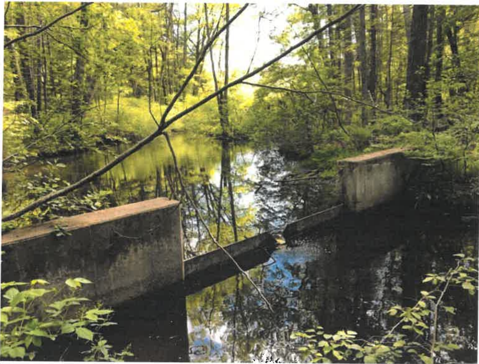
Photo 6 (06-06-18): Impoundment area with concrete and steel wall with a v-notch weir remotely located upstream of the Shore Road culvert. Two impoundments flow in series and then combine with the outflow from the nearby Dyer Pond Road culvert to discharge into the Shore Road culvert.
