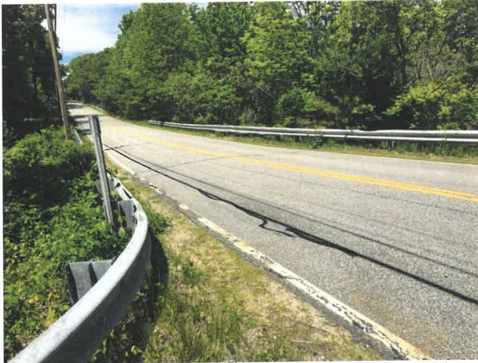
Photo 1 (06-06-18): Facing north at pavement surface of the Spurwink Avenue culvert crossing for the Jordan Pond outflow. Culvert crossing coincides with the pavement crack across the surface of Spurwink Avenue in the center of photo.
