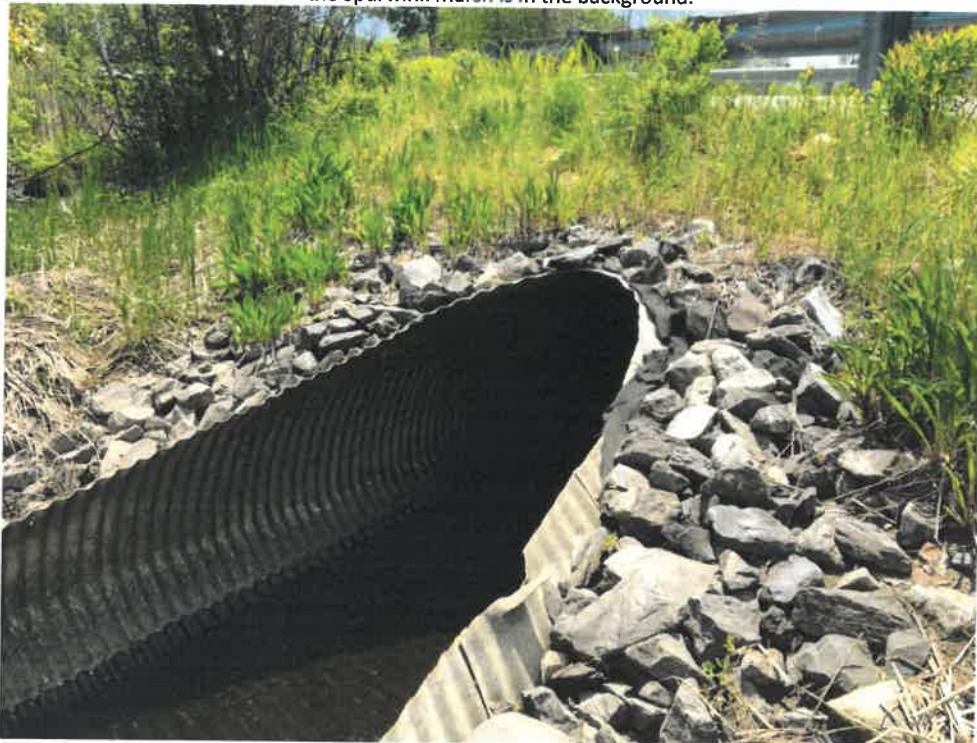
Photo 2 (06-06-18): Submerged inlet of 6-foot wide by 5-foot high corrugated aluminum elliptical pipe with flared end and rip rap headwall. Additional headwall rip rap should be added to the headwall.
