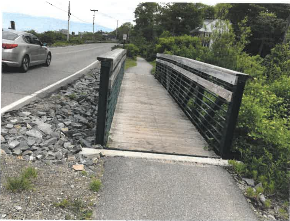
Photo 2 (06-06-18): Facing south at the Shore Road Path footbridge directly adjacent to the inlets of the three cross culverts.
