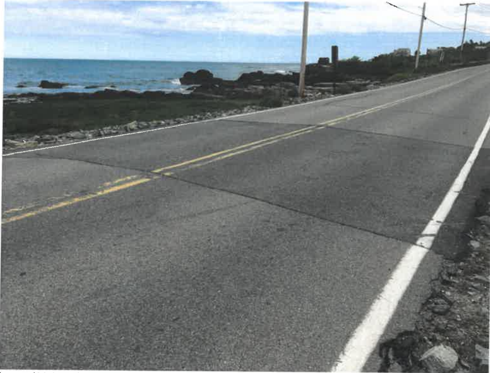
Photo 1 (06-06-18): Facing southeast at the Shore Road culvert crossing with Pond Cove in the background.
