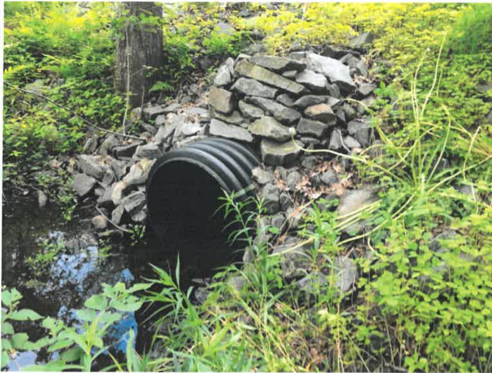
Photo 5 (06-06-18): Culvert outlet on west side of Spurwink Avenue with a rip rap headwall around the culvert.
