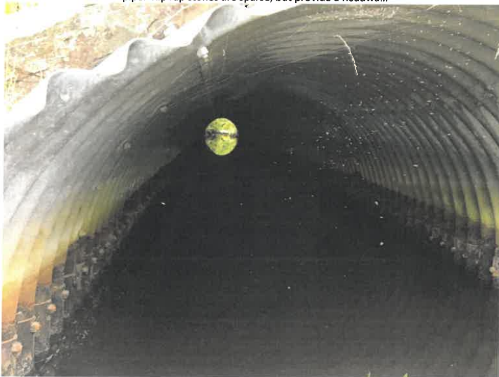
Photo 7 (06-06-18): Interior view of culvert from the outlet end on the west side of Route 77 toward the east side of Route 77 inlet. Corrosion evident along sidelines and invert of the pipe, however, the pipe alignment and integrity appear to visually be in good condition.
