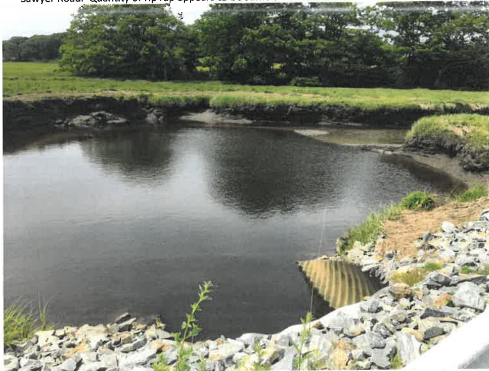
Photo 6 (06-06-18): Overhead view of culvert outlet and the widened area of the Spurwink River beyond the culvert outlet. The Spurwink River channel flows to the north (right hand side of this photo).
