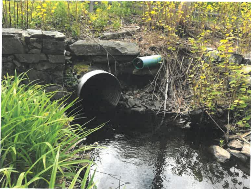
Photo 7 (06-06-18): Submerged outlet of culvert on the east side of Shore Road. Loose stones on headwall of outlet with smaller diameter green polyvinylchloride (pvc) pipe discharging well above the outlet invert elevation of the cross culvert.
