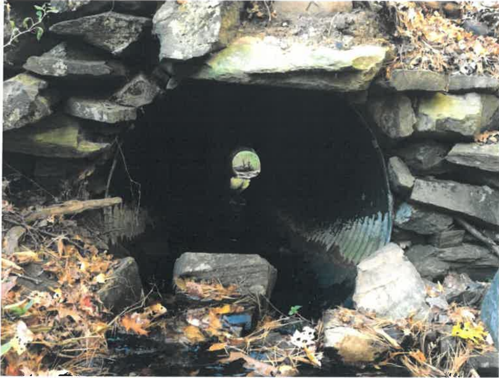
Photos 3 (10-22-18): Looking through the culvert from the inlet side, interior of the pipe appears visually to be in a degraded condition with the invert of the pipe clearly corroded.
