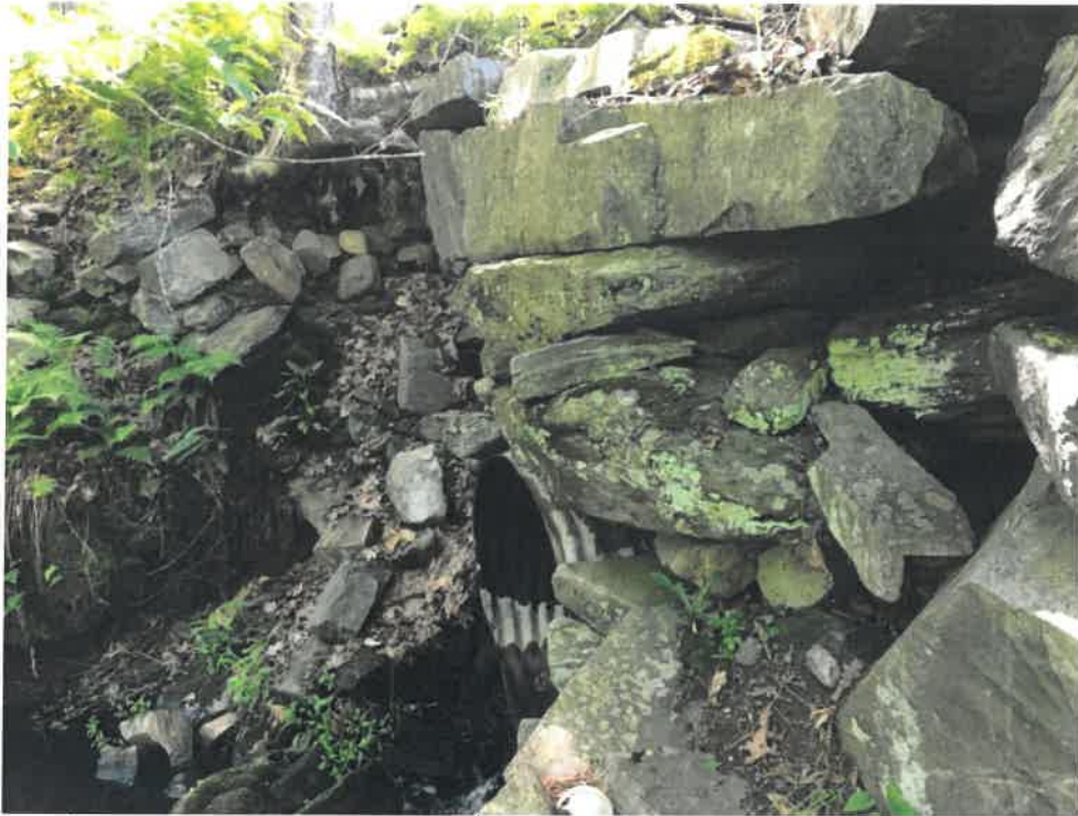
Photo 7 (06-06-18): Stone headwall at the outlet has deteriorated and has many loose and dislodged stones.
