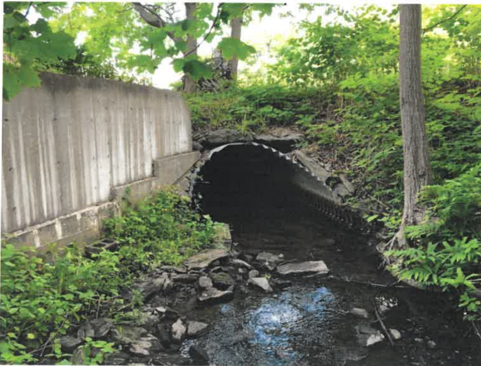
Photo 2 (06-06-18): Looking at the submerged Inlet of 8 foot, 2-inch-wide by 5 foot, 9-inch-high steel plate pipe arch cross pipe with concrete wingwall on the south side of Trout Brook. Inlet is on east side of Route 77.
