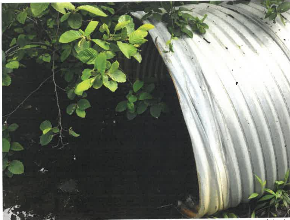
Photo 5 (06-06-18): Culvert outlet on east side of Spurwink Avenue is submerged within the corrugated aluminum pipe. Downstream vegetation obscured channel at the time of the photo.
