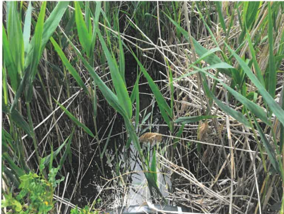
Photo 6 (06-06-18): Overhead view of culvert outlet and the vegetation beyond the culvert outlet.
