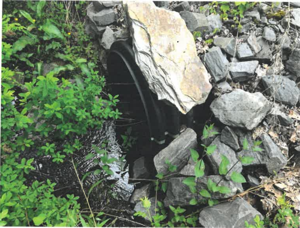
Photo 3 (06-06-18): Inlet of 30-inch High Density Polyethylene (HDPE) cross pipe with a rip rap creating a headwall and apron. Inlet is on the east side of Spurwink Avenue. Access to the culvert and the area around the inlet is relatively clear of vegetation.
