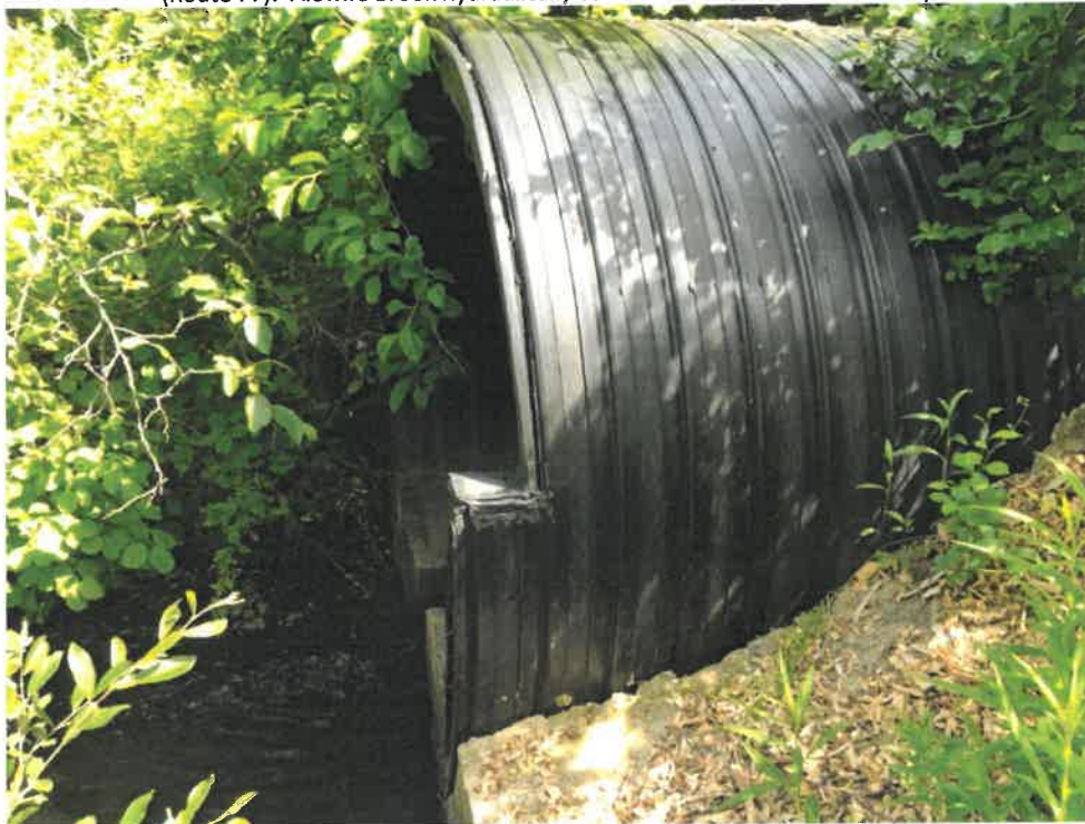
Photo 4 (06-20-18): Submerged outlet of culvert with slotted weir invert to slow the flow velocity through the pipe to allow fish passage. Culvert outlet is supported by concrete saddle.
