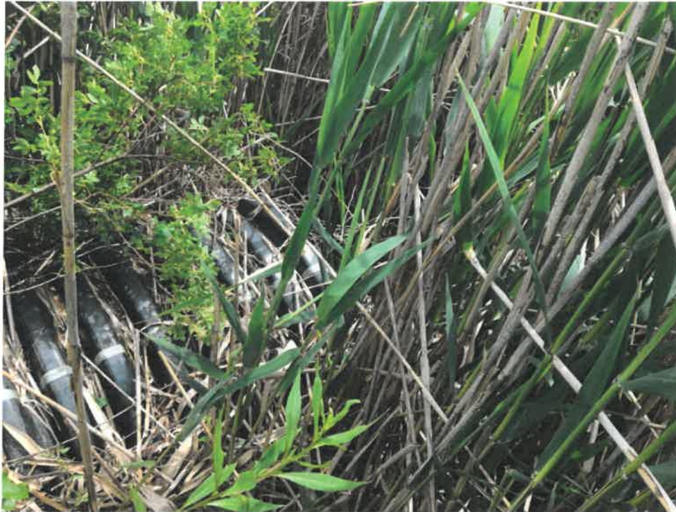
Photo 5 (06-06-18): Submerged outlet of the HDPE pipe on the west side of Sawyer Road. Thick vegetation around the end of the culvert could be better controlled with a rip rap apron.
