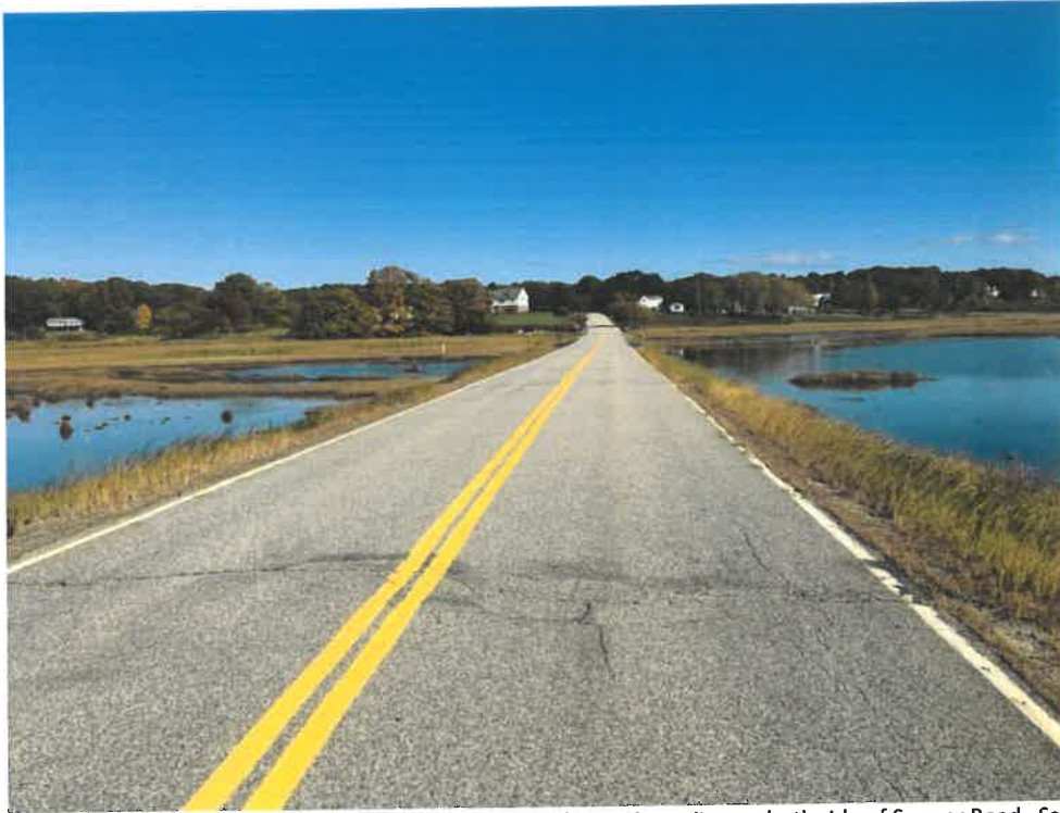
Photo 9 (10-22-18): Facing north during high tide of the Spurwink Marsh pooling on both side of Sawyer Road. Sawyer Road floods often during intense weather and tide events in the foreground of the photo as the road elevation is lower than at the culvert crossing which the inlet to the Spurwink River culvert is visible on the right side (east) of Sawyer Road.
