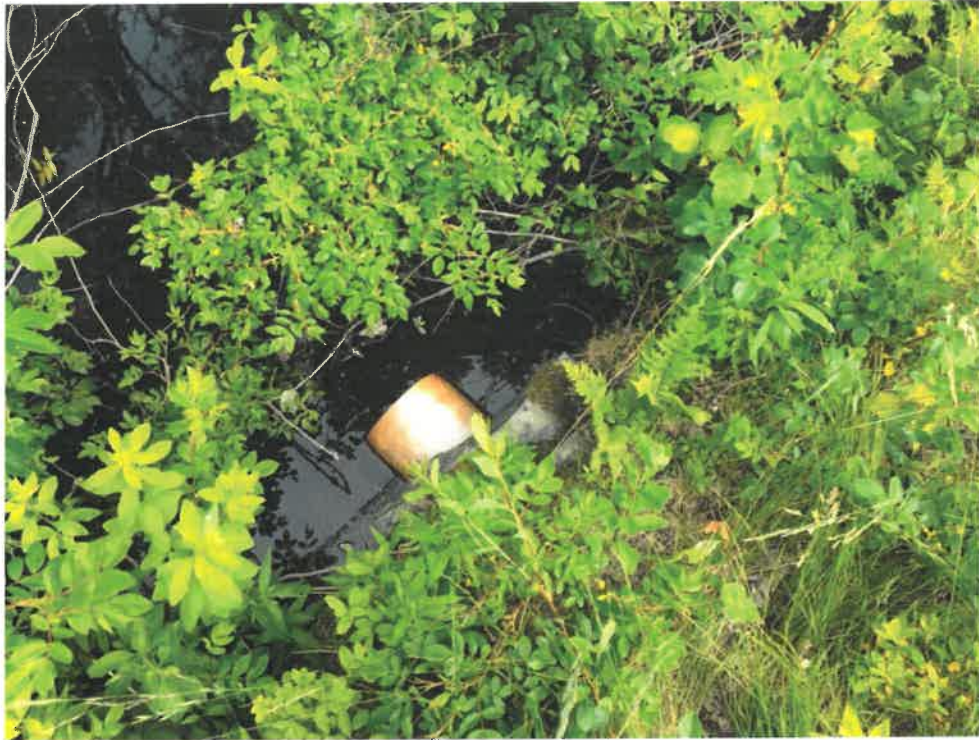
Photo 5 (06-20-18): Overhead view of submerged culvert outlet with a stone placed over the pipe to act as a headwall. Pipe is discolored due to years of exposure to sunlight.
