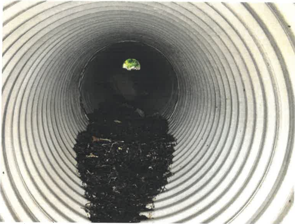
Photo 7 (06-06-18): Looking west at large rock and other ocean debris inside of northerly culvert. Being exposed directly to Casco Bay, ocean surges often push debris inside of these pipes creating an ongoing maintenance issue for the Town.
