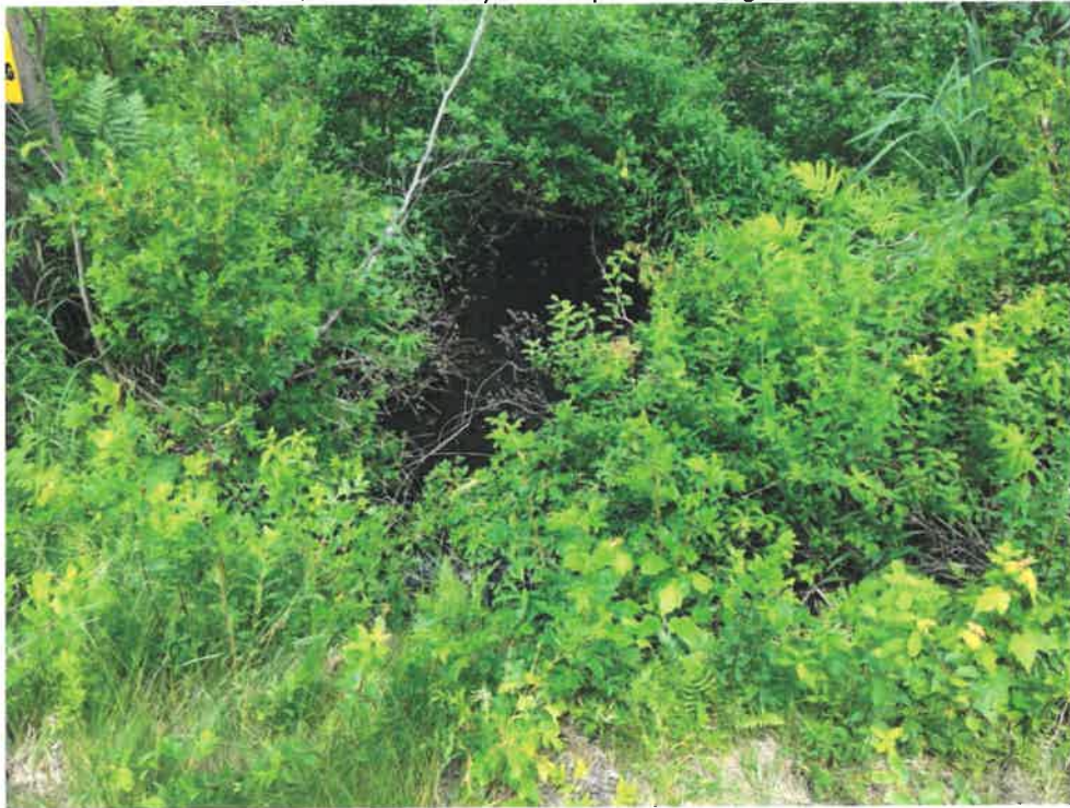
Photo 6 (06-20-18): Facing northeast at the downstream channel of the culvert outlet. Thick vegetation and likely deposited sediment within the channel create standing water with a very slow flow rate.
