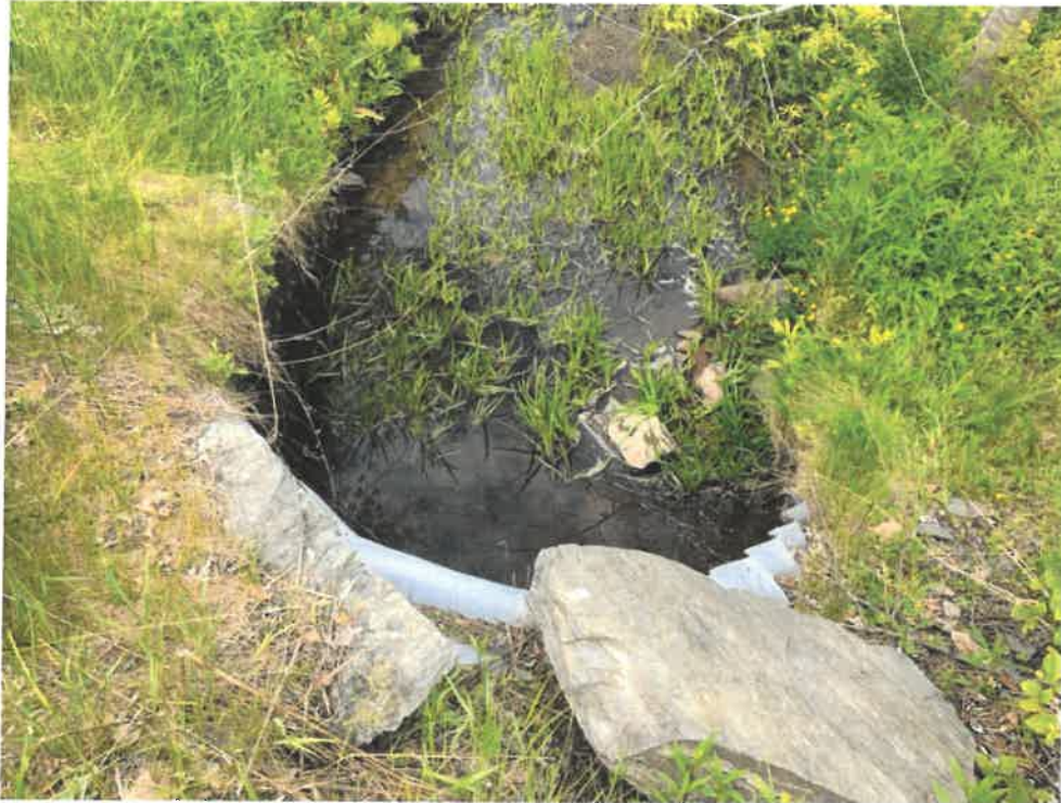
Photo 8 (06-06-18): Overhead view of culvert outlet with stones and vegetation in the outlet channel.
