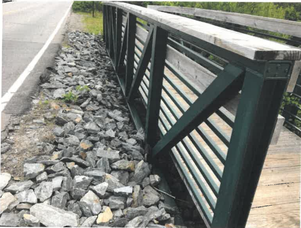
Photo 3 (06-06-18): Facing South. The presence of the footbridge directly over the culvert inlets and stone rip rap make inlet maintenance a challenge
