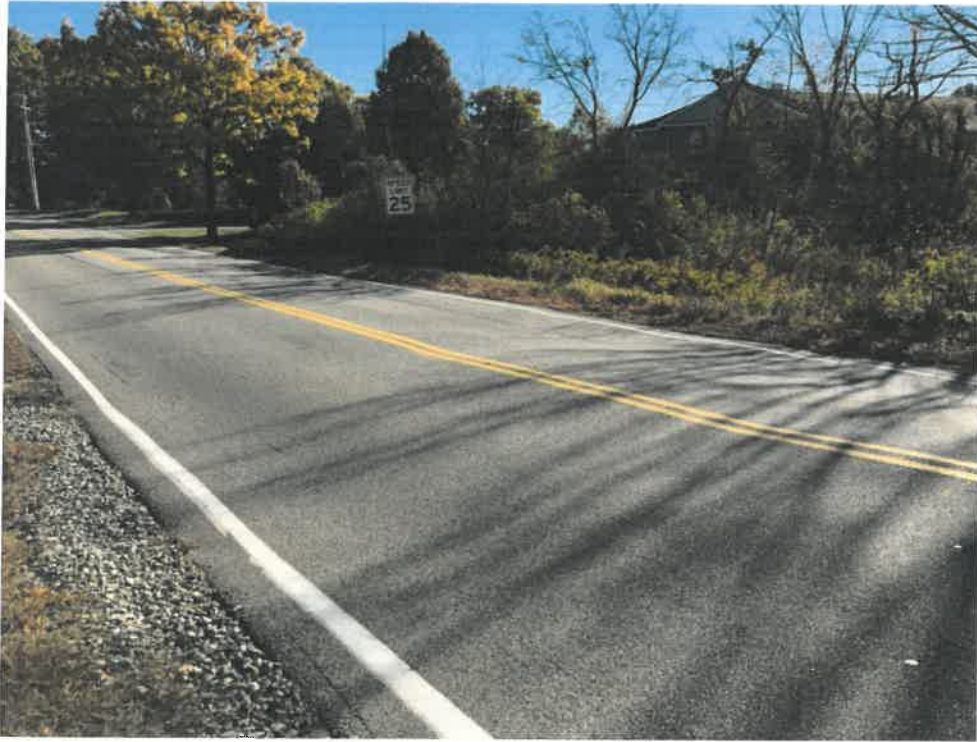
Photo 1 (10-22-18): Facing east at Scott Dyer Road at the Willow Brook culverts crossing.
