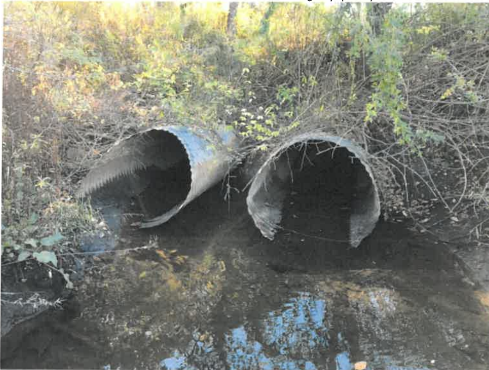
Photo 2 (10-22-18): Inlets of the two, 48-inch wide by 36-inch tall corrugated aluminum pipes located northerly of the sanitary sewer crossing embankment. Inverts to both pipes are corroded and in decay.
