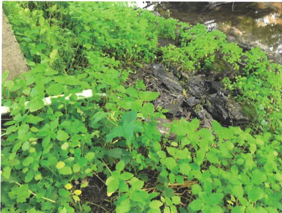
Photo 5 (06-06-18): Facing west at the east end of the concrete wingwall on the south side of the culvert inlet. Small diameter white pvc pipe is conveying groundwater flow directly into Trout Brook despite being a relatively dry weather period. Trout Brook receives surface flow and groundwater flow from residential neighborhoods and other developed areas in close proximity to the stream.
