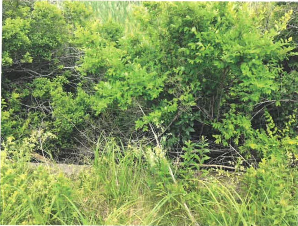
Photo 3 (06-20-18): Facing east at granite headwall of the culvert inlet with thick vegetation blocking the inlet area of the culvert. Providing a rip rap apron at the inlet would control vegetation from blocking the inlet.
