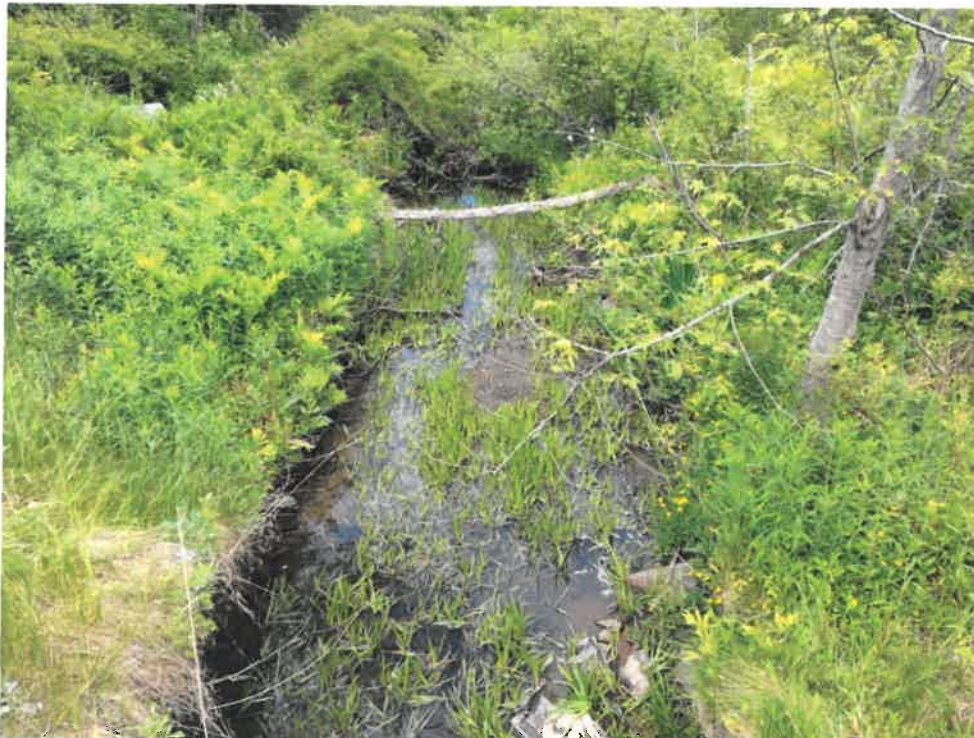
Photo 9 (06-06-18): Looking further downstream at the outlet of the steel plate pipe arch cross pipe. Vegetation and sediment deposits are present within this channel.
