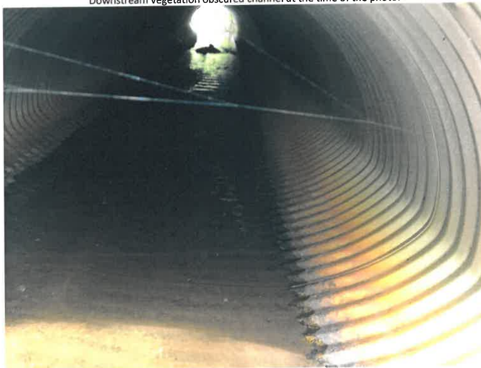
Photo 6 (06-06-18): Interior view of culvert taken from outlet to the inlet of culvert. Some corrosion visible along invert of pipe, however, the culvert appears visibly to be in good condition.
