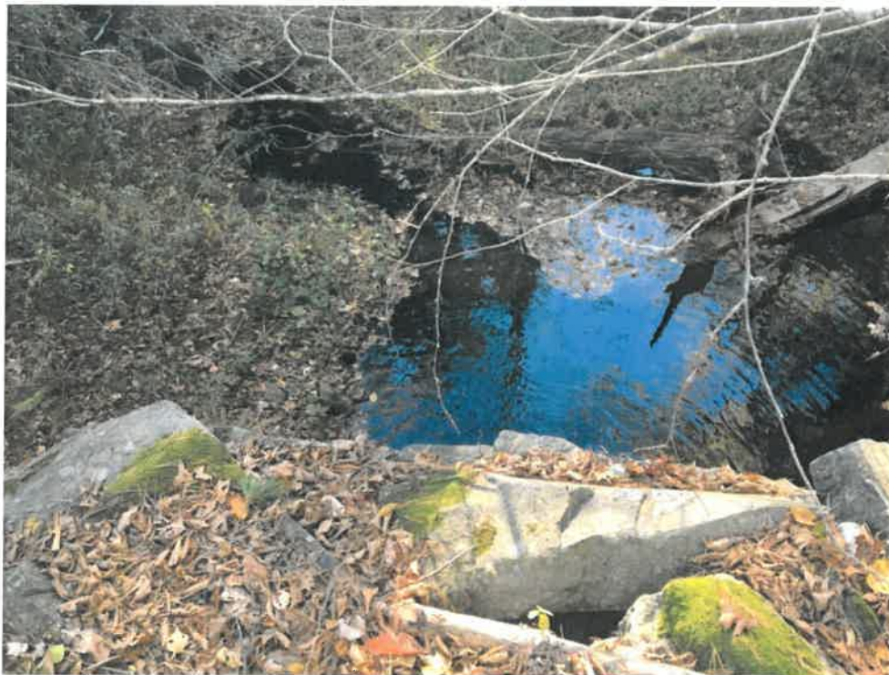
Photo 8 (10-22-18): Overhead view of culvert outlet with loose stones in the stone headwall.
