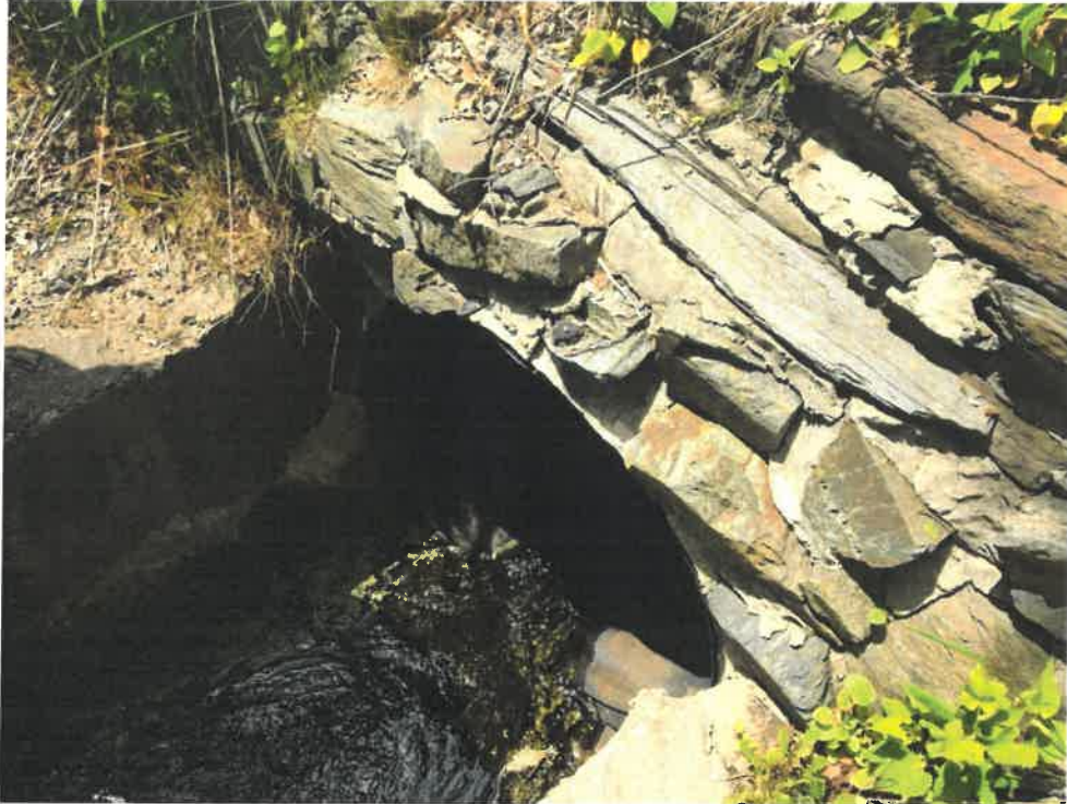
Photos 5 (06-06-18): 36-inch Corrugated Metal Pipe (CMP) Culvert inlet on south side of Spurwink Avenue. Pipe transitions into a 36-High Density Polypropylene (HDPE) under roadway. Grouted stone provides a headwall for the culvert inlet.
