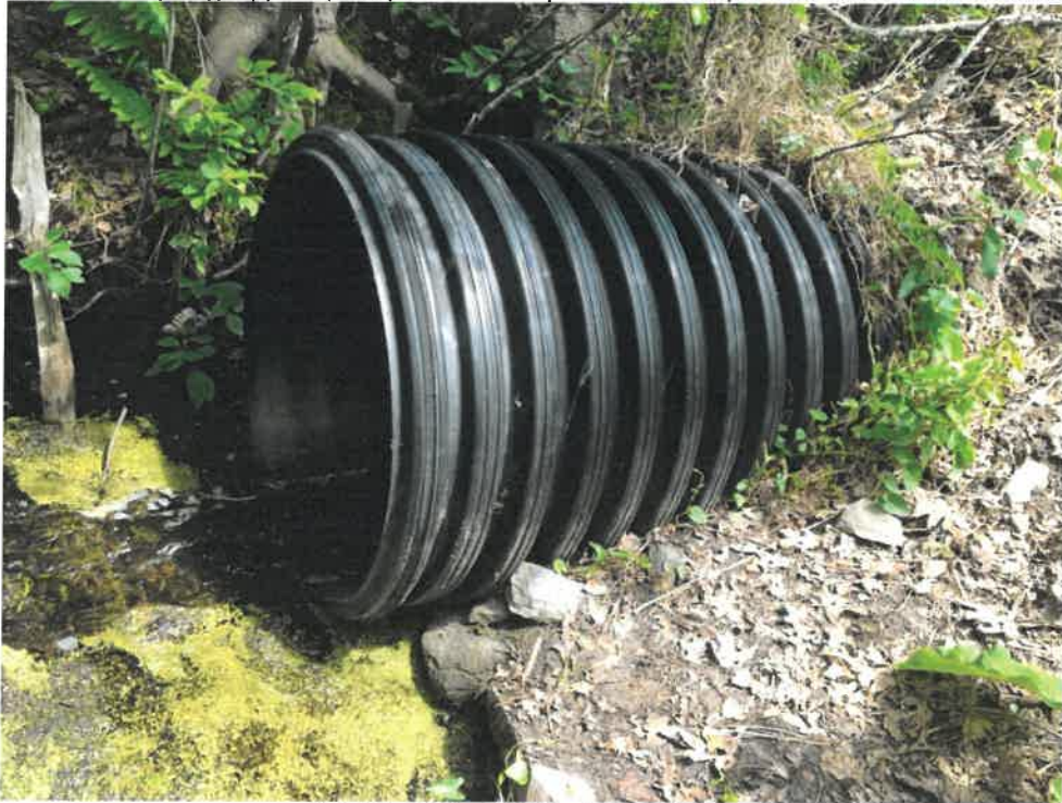
Photo 6 (06-06-18): Looking at the outlet of the 36-inch HDPE culvert on the north side of Spurwink Avenue. No formal headwall or apron at the outlet.
