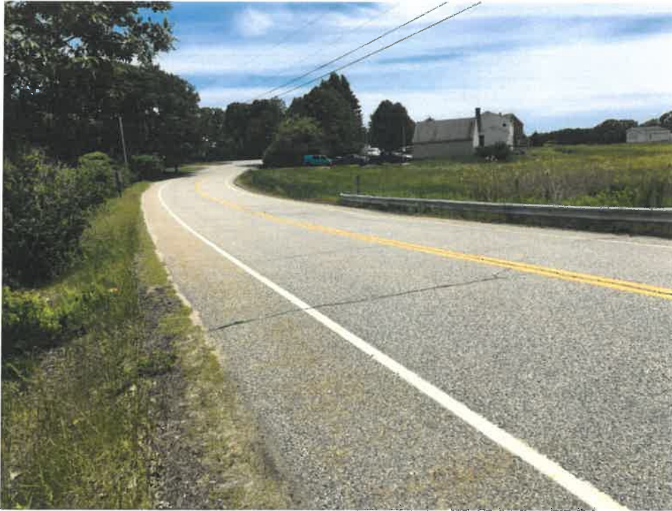
Photo 1 (06-20-18): Facing south Sawyer Road crossing of the culvert. Crack on surface of the road may be due to the presence of culvert.
