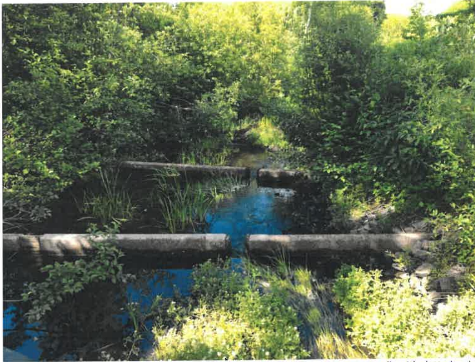
Photo 7 (06-20-18): Downstream channel of the culvert outlet flow with two concrete weir walls with slotted weirs to control elevation and flow from the culverts to dissipates energy of the outfall and reduce the velocity of the outflow to the receiving channel. The weirs also create pool areas within the channel.
