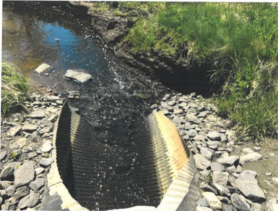
Photo 7 (06-06-18): Overhead view of culvert outlet with stones in and beyond the flared apron area. Headwall stones around the culvert appear to be depleted of rip rap layers and should be replenished.
