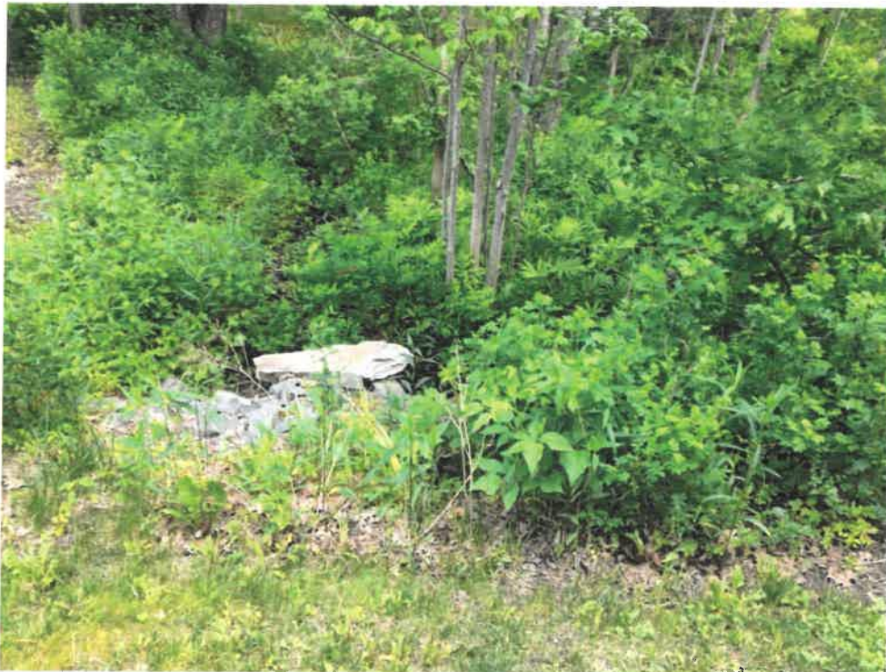
Photo 4 (06-06-18): Facing east at the inlet of 30-inch HDPE cross pipe and the vegetated channel upstream of the culvert crossing.
