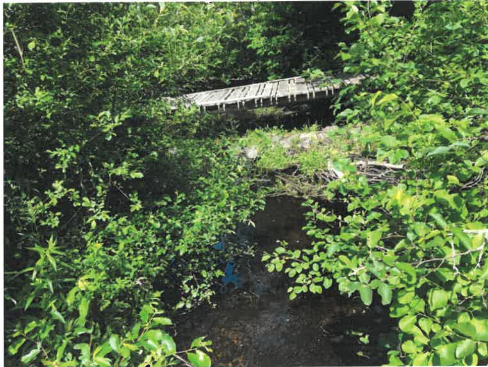
Photo 8 (06-20-18): Downstream view of Alewife Brook from outlet area of the culvert. Stone berm is upstream of a wooden footbridge crossing over the stream in the background of the photo.
