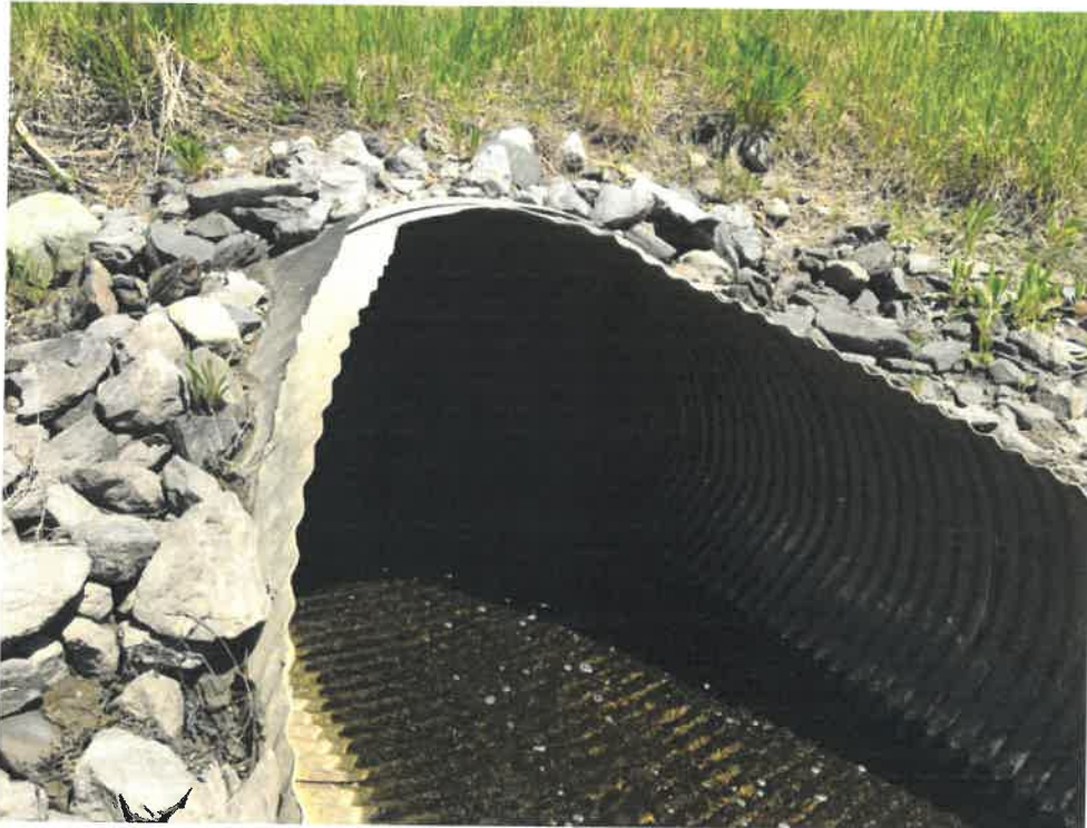
Photo 5 (06-06-18): Submerged outlet of the aluminum elliptical pipe with flared end and rip rap headwall. Additional rip rap would be desirable to bolster the area around the culvert.
