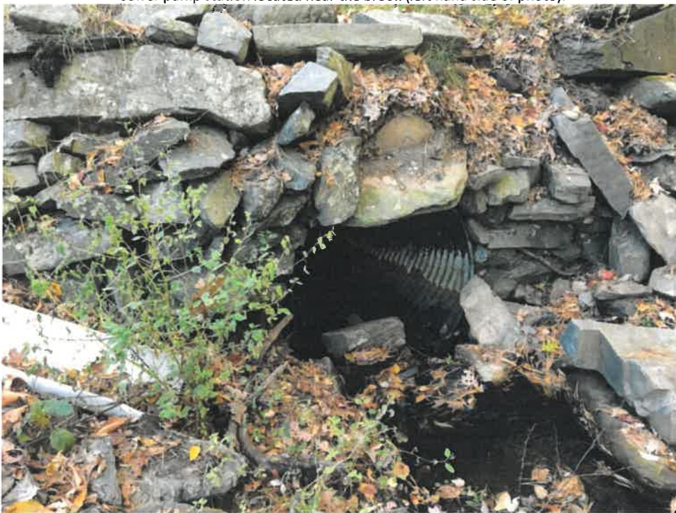
Photo 2 (10-22-18): Submerged inlet of 48-inch corrugated metal pipe with corroded invert and various stones blocking the inlet from reaching full flow capacity. The stone headwall needs to be reset.
