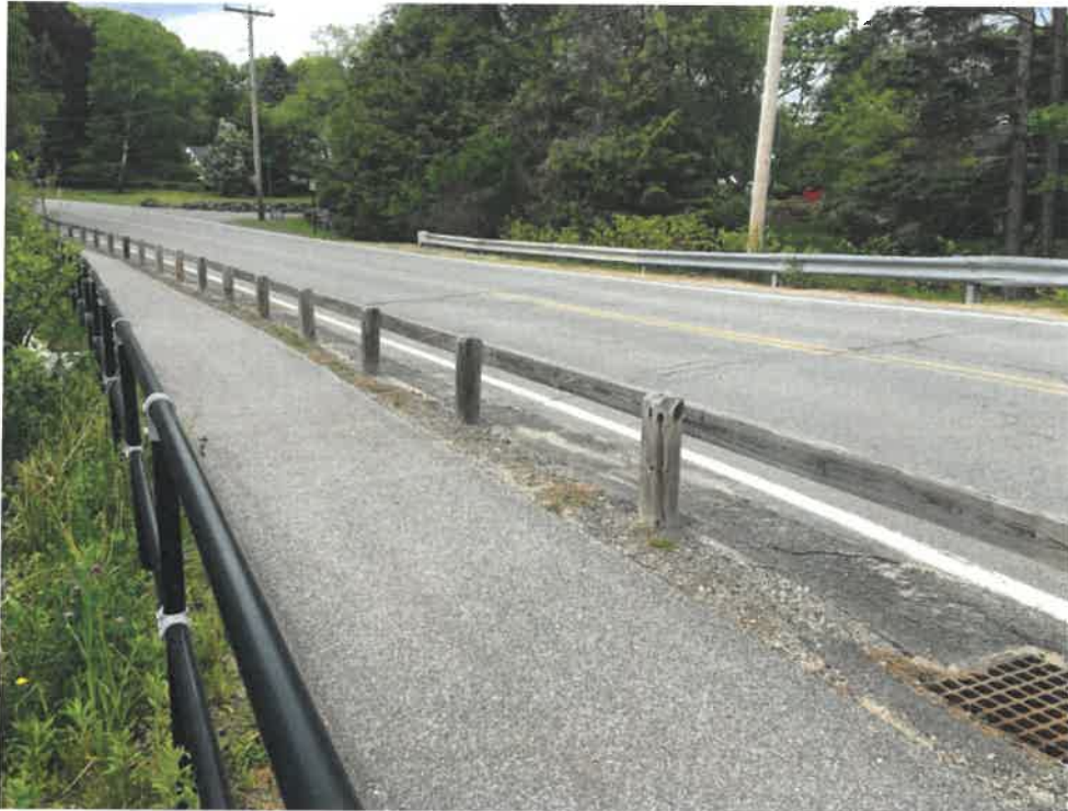
Photo 1 (06-06-18): Facing northeast at Shore Road crossing of the Dyer Pond outflow. Culvert crossing coincides with the pavement crack across the surface of Shore Road.
