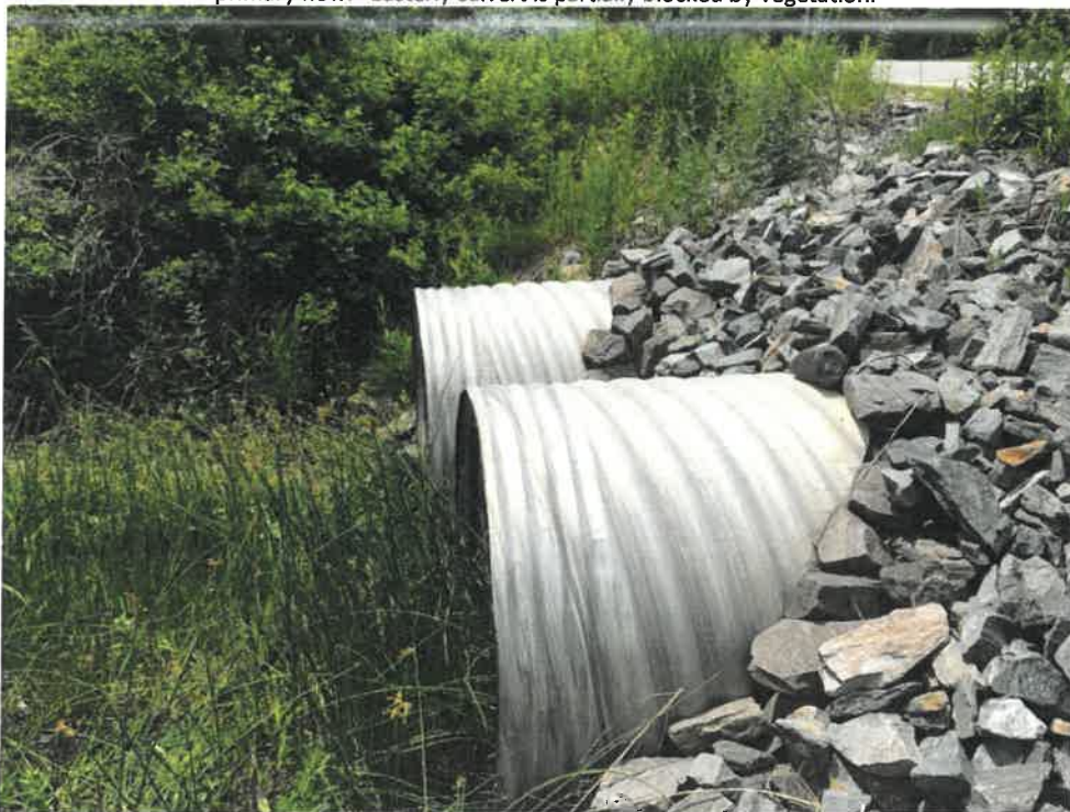
Photo 6 (06-20-18): Culvert outlet discharge of Willow Brook on the south side of Scott Dyer Road. Some limited vegetation removal and rip rap at the end of the easterly pipe would ensure that its capacity is not compromised by additional vegetation growth.
