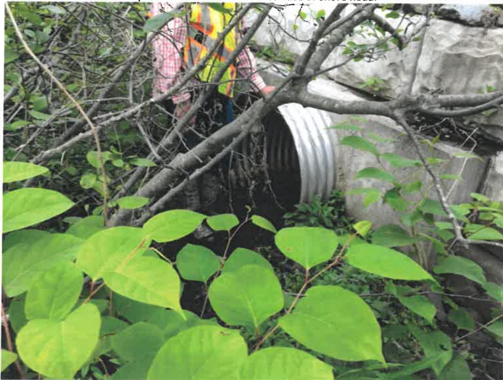
Photo 2 (06-06-18): Inlet of 36-inch corrugated aluminum cross pipe with a cast-in-place concrete collar and base set within a large concrete block "Stonestrong" retaining wall. Inlet is on the west side of Shore Road.
