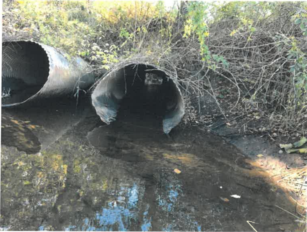
Photos 3 (10-22-18): Looking down the barrel of the westerly inlet of the two Inlet culverts. Culverts' inlet invert has rusted away and the pipes are in poor condition.
