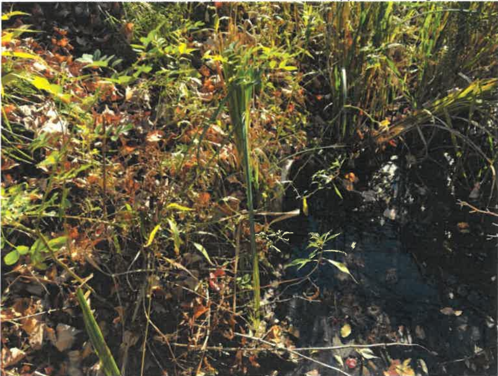
Photo 2 (10-22-18): Submerged inlet of 10-inch polyvinylchloride (pvc) culvert is barely visible due to the standing water and the vegetation surrounding the pipe. No rip rap apron or headwall. Pipe is very shallow and flat which compromises its capacity.
