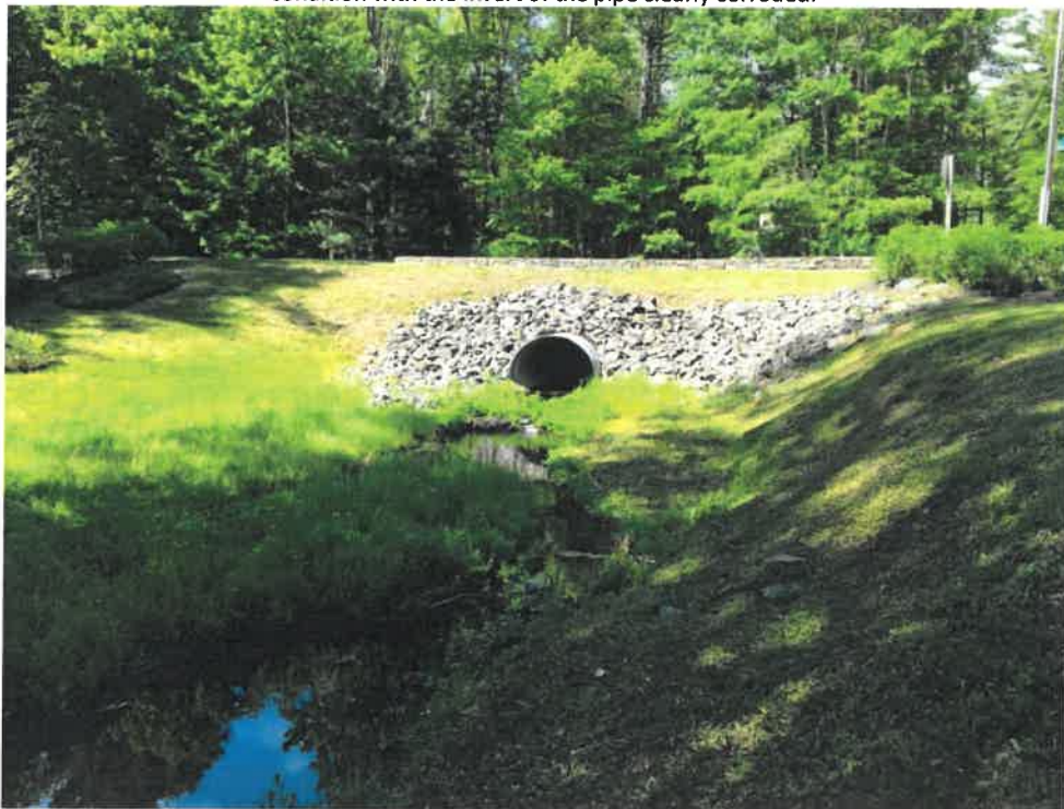
Photo 4 (06-06-18): Facing northwest from the Mitchell Road culvert toward the 3-feet tall by 4-feet wide elliptical culvert under nearby Hobstone Road with channel of the Pond Cove Brook upstream of the Mitchell Road culvert inlet.
