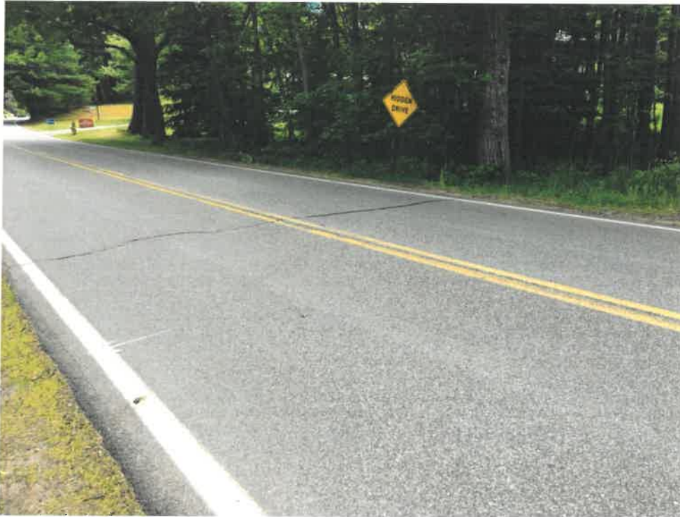
Photo 1 (06-06-18): Facing south at pavement surface of the Spurwink Avenue culvert crossing for an unnamed tributary to Trout Brook. Culvert crossing coincides with the pavement crack across the surface of Spurwink Avenue in the center of photo.
