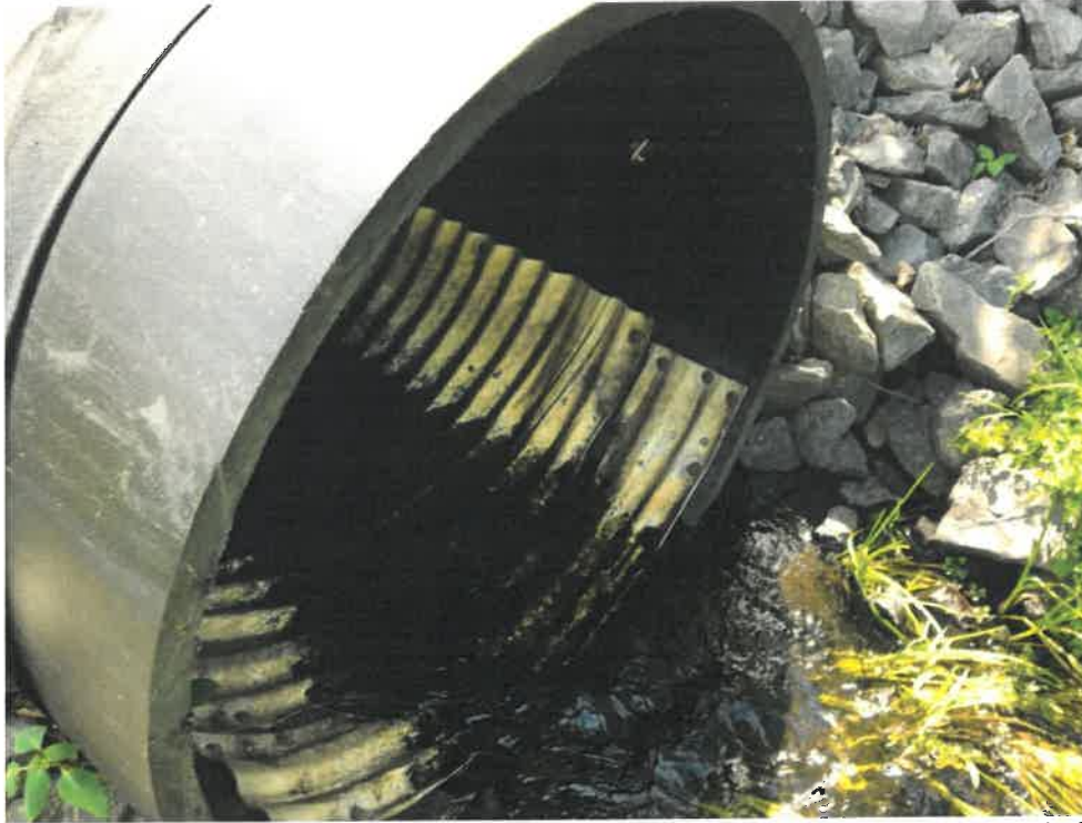
Photo 5 (06-20-18): Submerged outlet of main flow carrying culvert with corrugated metal pipe invert to slow the flow velocity through the pipe to allow fish passage.
