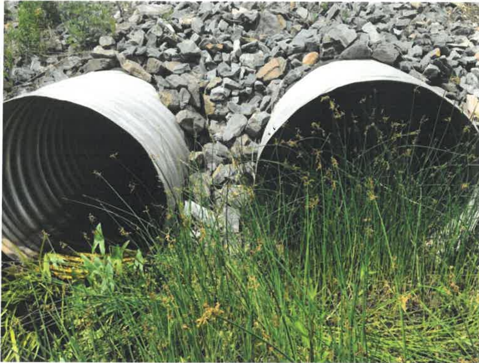
Photo 5 (06-20-18): Outlet of culverts on the south side of Scott Dyer Road. Westerly (left) pipe is set lower and carries the primary flow. Easterly culvert is partially blocked by vegetation.
