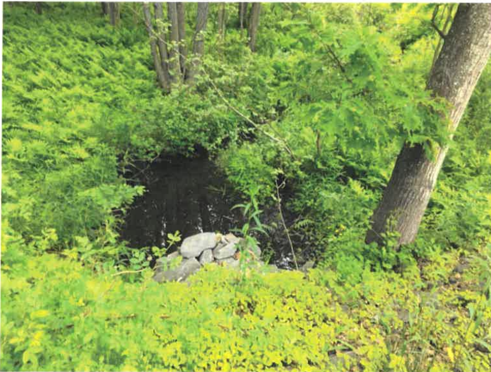
Photo 6 (06-06-18): Facing west at the stone headwall for the outlet of 30-inch HDPE cross pipe and the channel downstream of the culvert crossing. The downstream channel turns to the north (i.e., the right in this photo) as it approached the vegetation beyond the visible pool of water beyond the outlet of the culvert.
