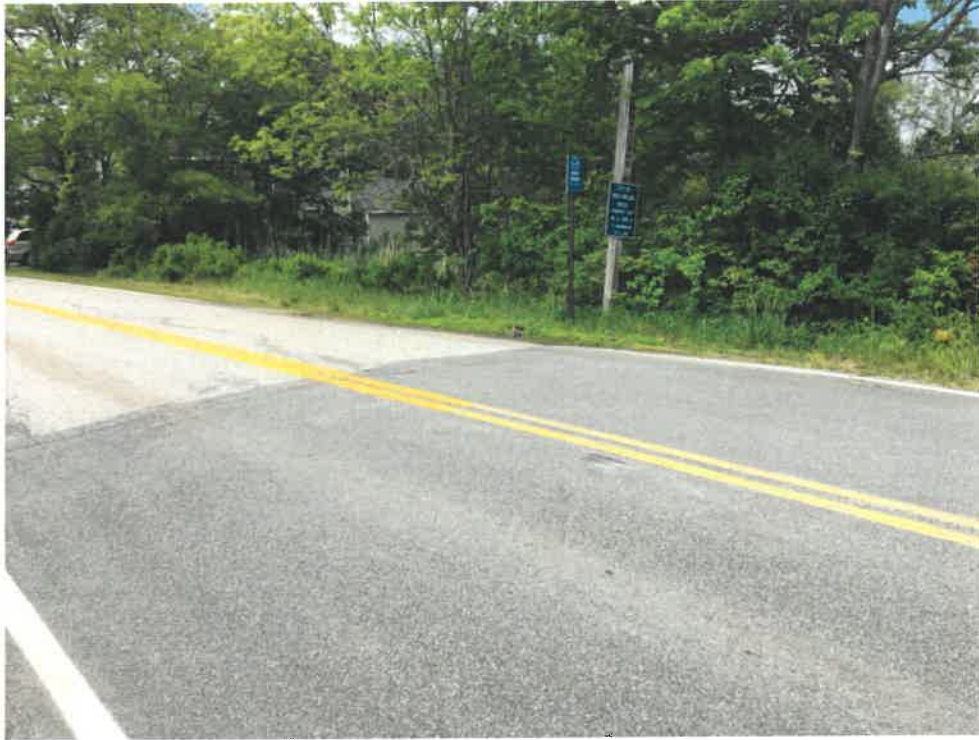
Photo 1 (06-06-18): Facing northeasterly at Spurwink Avenue crossing with Trout Brook which is an Urban Impaired Stream. Culvert crossing coincides with the pavement crack and change in pavement seam (which is also the South Portland municipal boundary) across the surface of Spurwink Avenue. Smaller blue sign indicates that the culvert is in the Trout Brook Watershed.
