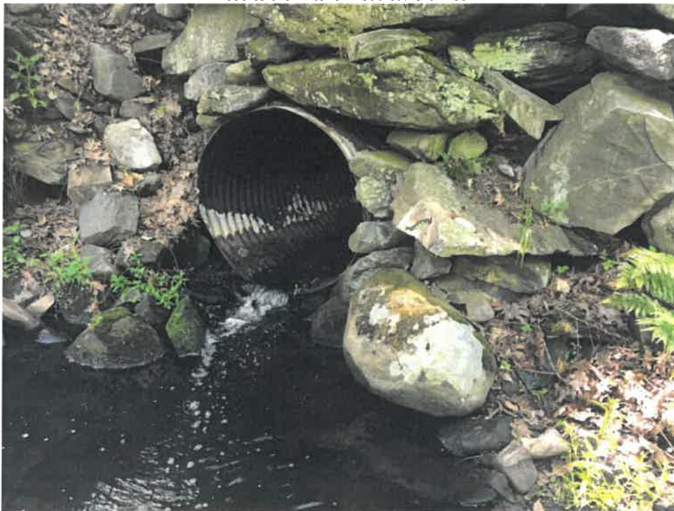
Photo 6 (06-06-18): Hanging outlet of the aluminum elliptical pipe with flared end and rip rap headwall. Additional rip rap would be desirable to bolster the area around the culvert.
