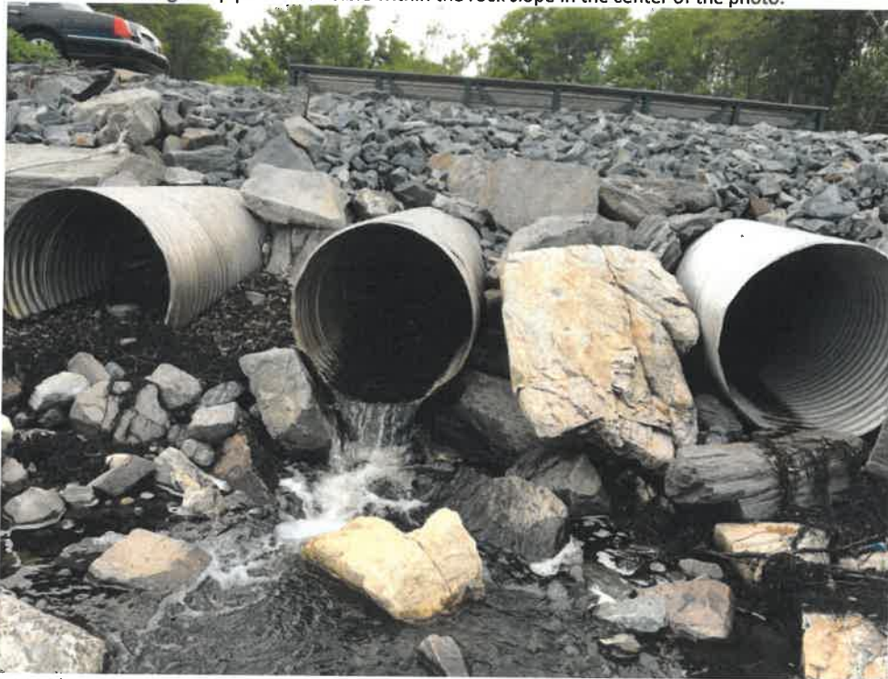
Photo 6 (06-06-18): Looking east at hanging outlet of the three, 36-inch aluminum corrugated pipe outlets on the west side of Shore Road. Seaweed and other debris frequently compromise the culverts' capacity as exemplified by only the center culvert flowing freely despite all three culverts being installed at roughly the same elevations.
