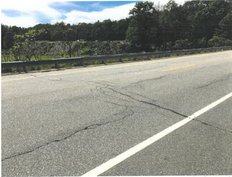
Photo 1 (06-20-18): Facing west at Ocean House Road (Route 77) crossing of Alewife Brook. Culvert location coincides with the crack across the pavement surface. Culvert is located relatively deep in relation to the road surface elevation with a steep roadway embankment.
