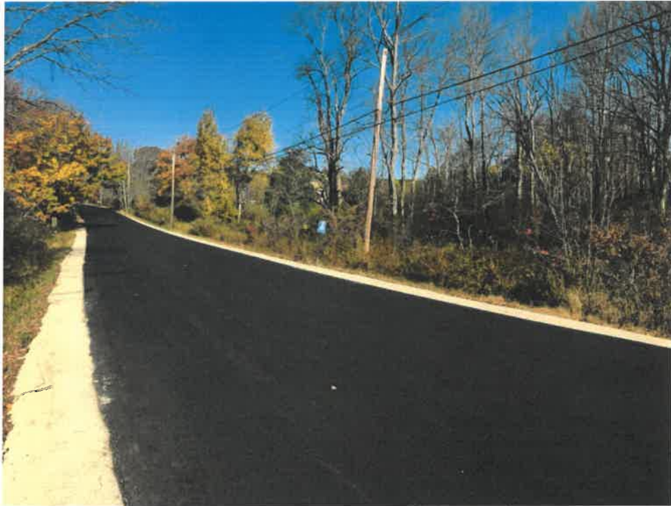
Photo 1 (10-22-18): Facing north at Eastman Road crossing of Trout Brook. Blue sign indicates that the culvert is within the Trout Brook Watershed which is an Urban Impaired Stream. Road freshly paved with new gravel shoulders.
