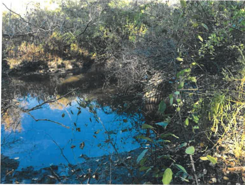
Photo 7 (10-22-18): Downstream channel of Willow Brook from the culvert outlet flow has marine sediment deposits from the tidal marsh.
