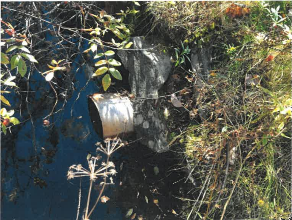
Photo 4 (10-22-18): Submerged outlet of culvert on the east side of Eastman Road. No rip rap apron has been provided. Area around the outlet has thick vegetation and standing water and is not draining well.
