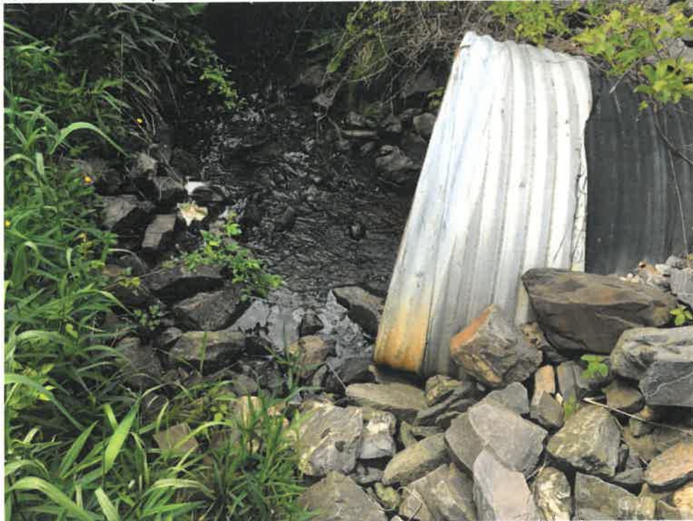
Photo 2 (06-06-18): Inlet of 60-inches wide by 44-inches tall corrugated aluminum elliptical cross pipe with rip rap apron and headwall. Flow curls into culvert abruptly after flowing southerly along and parallel to Spurwink Avenue.
