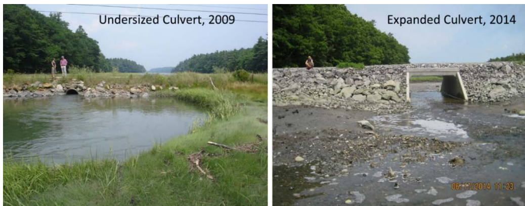
Figure 7. Culvert at northern end of Long Marsh, prior to and after the 2014 restoration.
