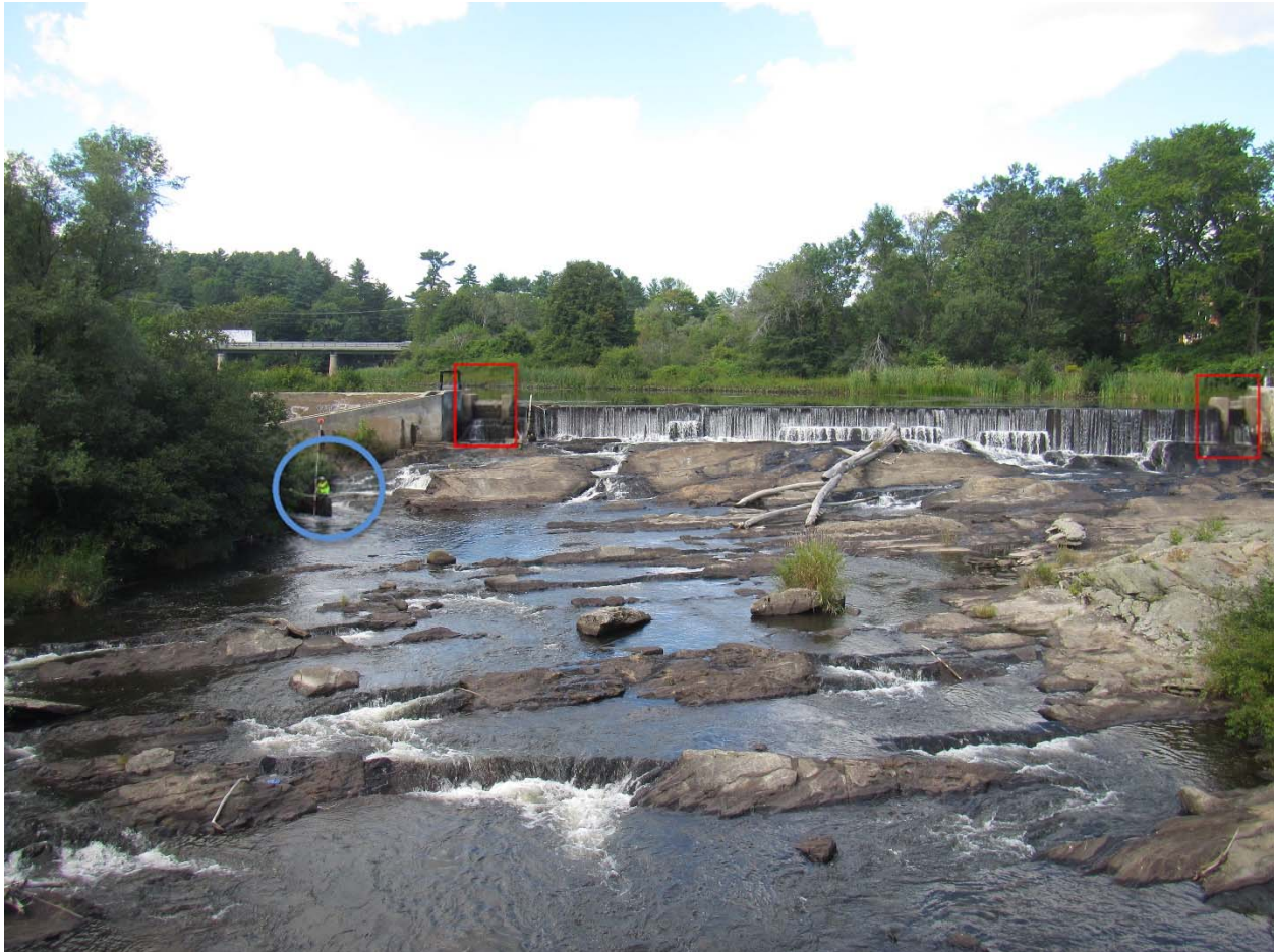
Figure 4: View looking upstream at Bridge Street Dam. Stop log weirs are indicated within the red squares and fishway entrance is indicated with a blue circle. Note surveyor for size. Flow direction is toward viewer.
