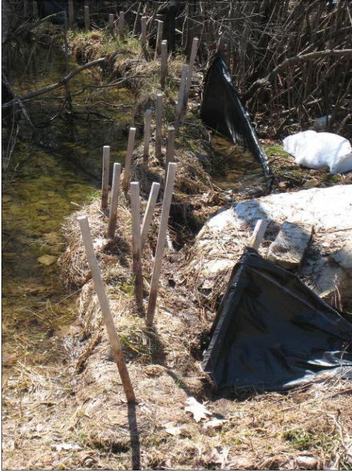
A collapsed silt fence observed at a construction site in the Sabbathday Lake Watershed.
