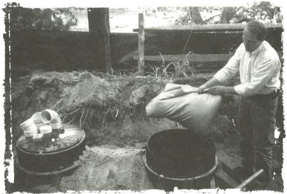
Jim Gray of SeptiTech installs a new septic system technology at Brighams Cove, Casco Bay. Seven overboard discharges were removed, which will allow this cove to be opened for shellfishing.
